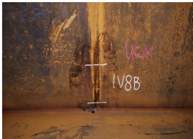
Photo #2: Typical vertical spot from bottom (0-150mm)
