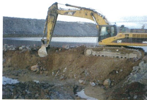
(08-26-2012) NP1 - 1st Breach 3
