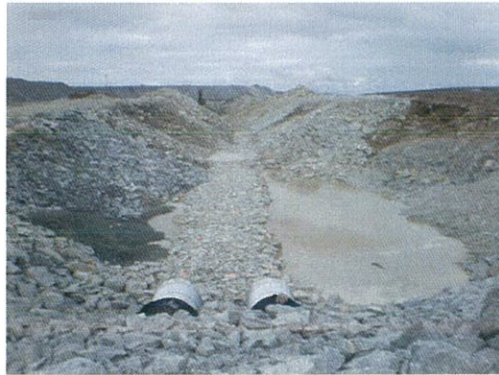
(08-26-2012) NP1 - 1st Breach 9
