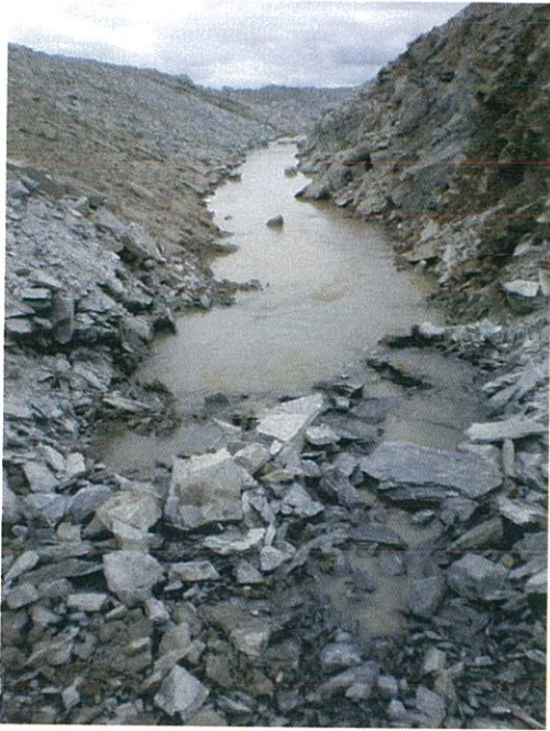
(08-26-2012) NP1 - 1st Breach 11
