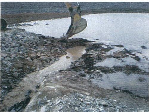
(09-17-2012)NP1 – 3rd Breach 1
