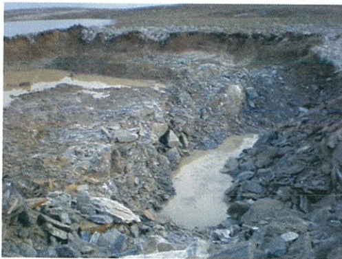
(08-26-2012) NP1 - 1st Breach 1
