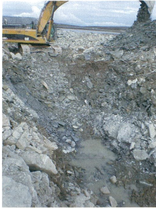
(08-26-2012) NP1 - 1st Breach 8
