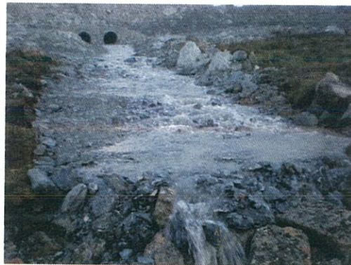
(08-27-2012) NP1- 1st Breach 14
