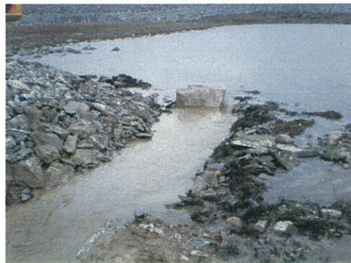
(09-17-2012)NP1 – 3rd Breach 4
