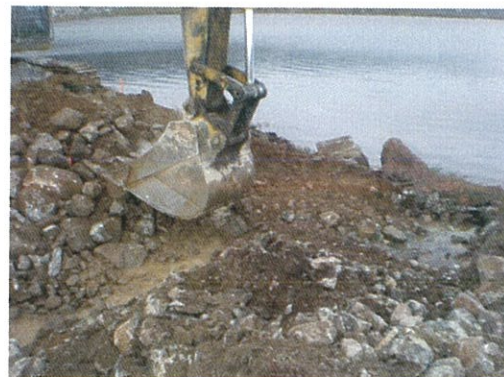
(08-26-2012) NP1 - 1st Breach 4
