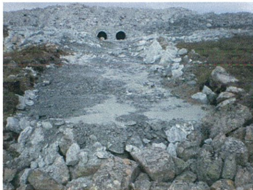
(08-26-2012) NP1 - 1st Breach 10
