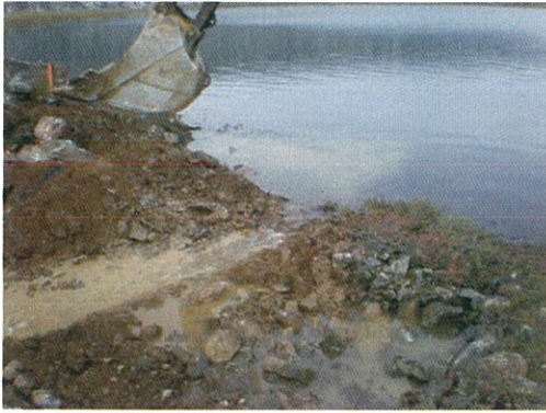
(08-26-2012) NP1 - 1st Breach 5
