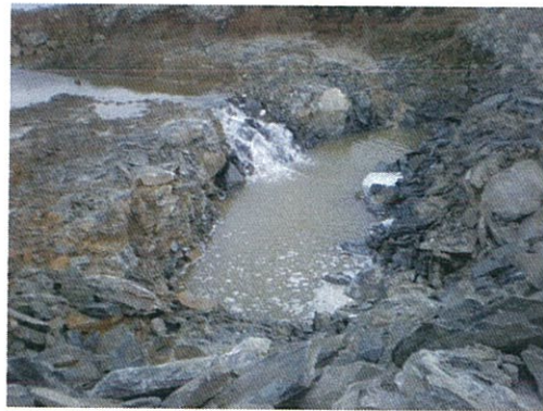
(08-27-2012) NP1- 1st Breach 13
