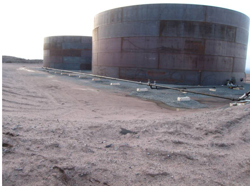
PHOTOGRAPH 7 – Baker Lake Tank Farm
