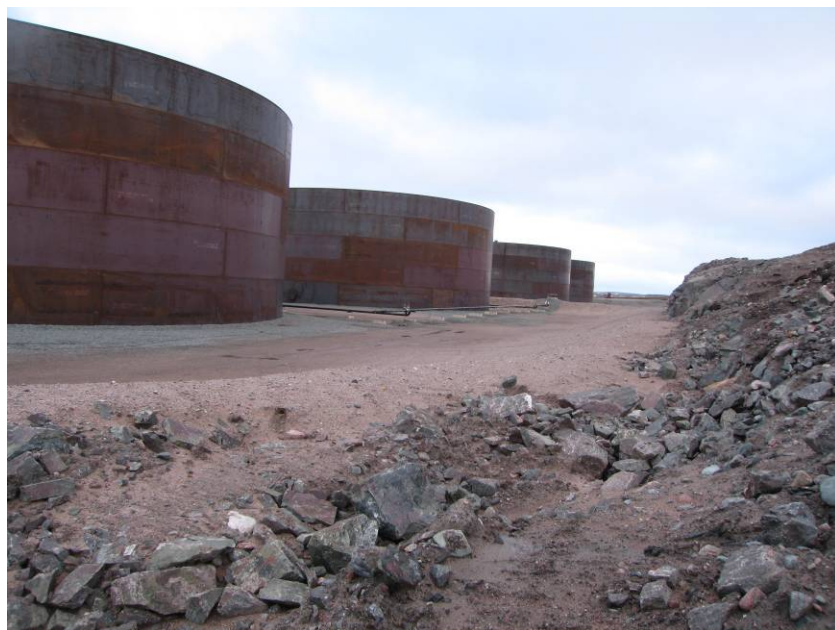
PHOTOGRAPH 8 – Baker Lake Tank Farm
