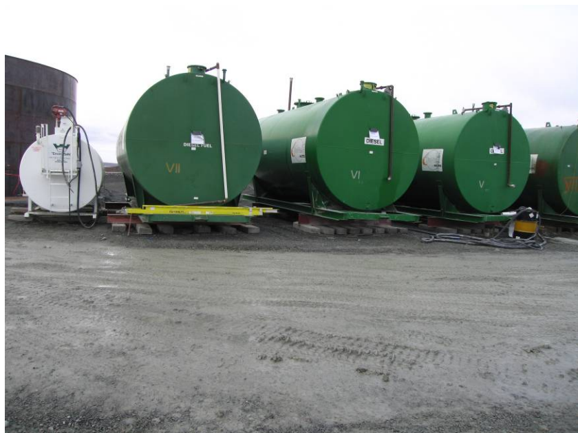
PHOTOGRAPH 5 – Meadowbank Tank Farm
