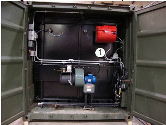
Primary Chamber Burner Flexible lines
