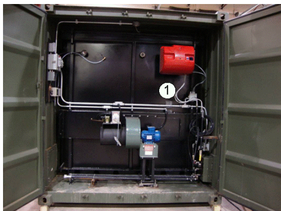
Primary Chamber Burner Flexible lines (Item # 1 Above)
