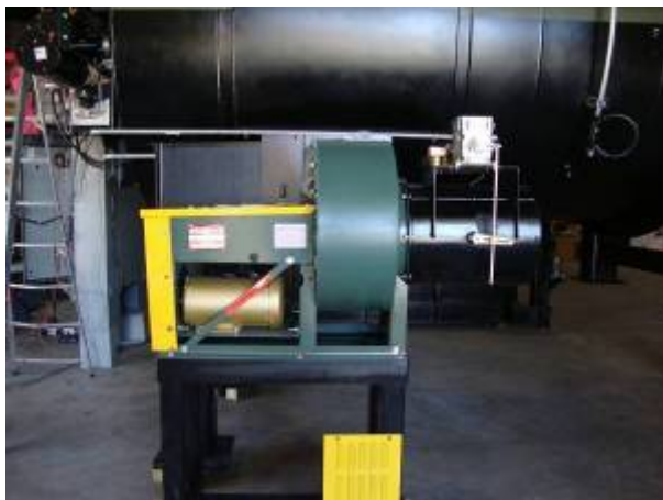
Secondary Chamber Blower
