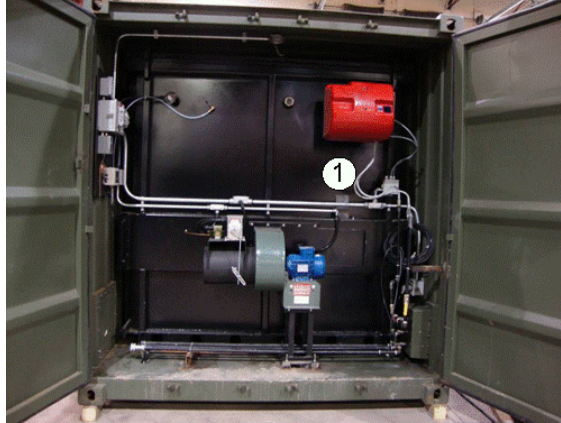
Primary Chamber Burner Flexible lines
