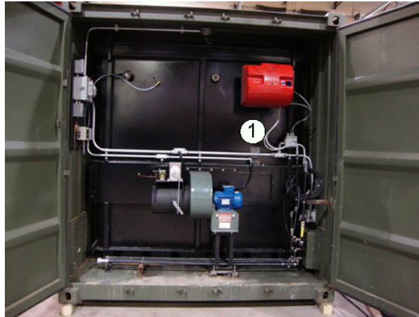
Primary Chamber Burner Flexible lines
