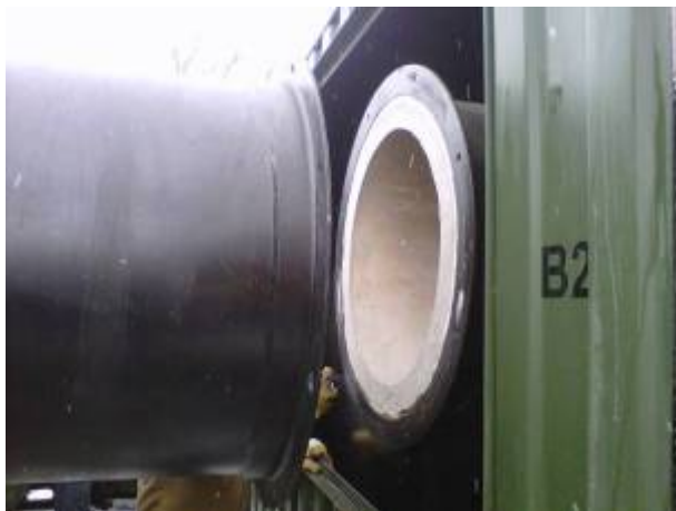
Gasket NOT installed
