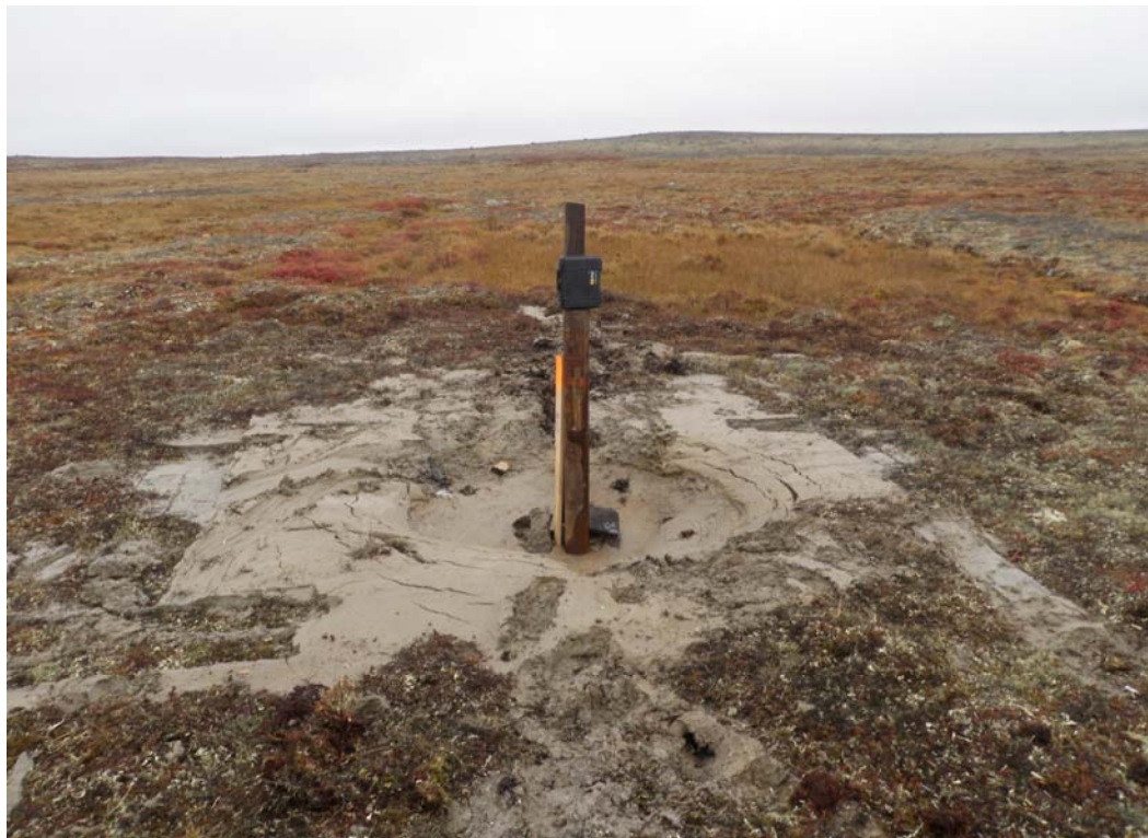
PHOTOGRAPH 3: Looking at GT11-05 Thermistor installation.
