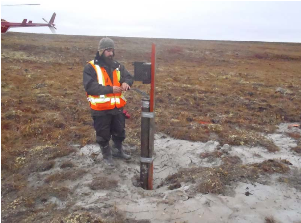
PHOTOGRAPH 5: Looking E at GT11-12 Thermistor installation.
