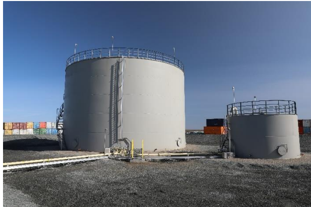
Photo 22. Fuel Tank Farm#1.
