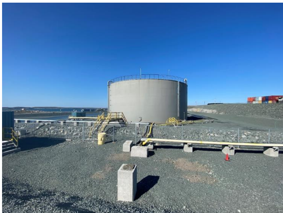
Photo 2: Fuel Farm 2 and Secondary Containment
