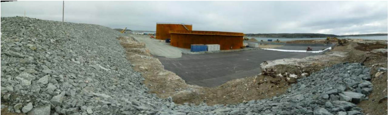
Photograph 3: Itivia Site, Tank #1 and #2 Storage Area from North Corner, Looking South (22 September 2017)
