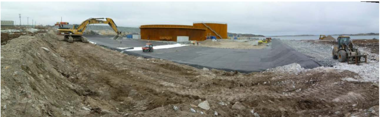
Photograph 4: Itivia Site, Tank #1 and #2 Storage Area from West Corner, Looking East (22 September 2017)
