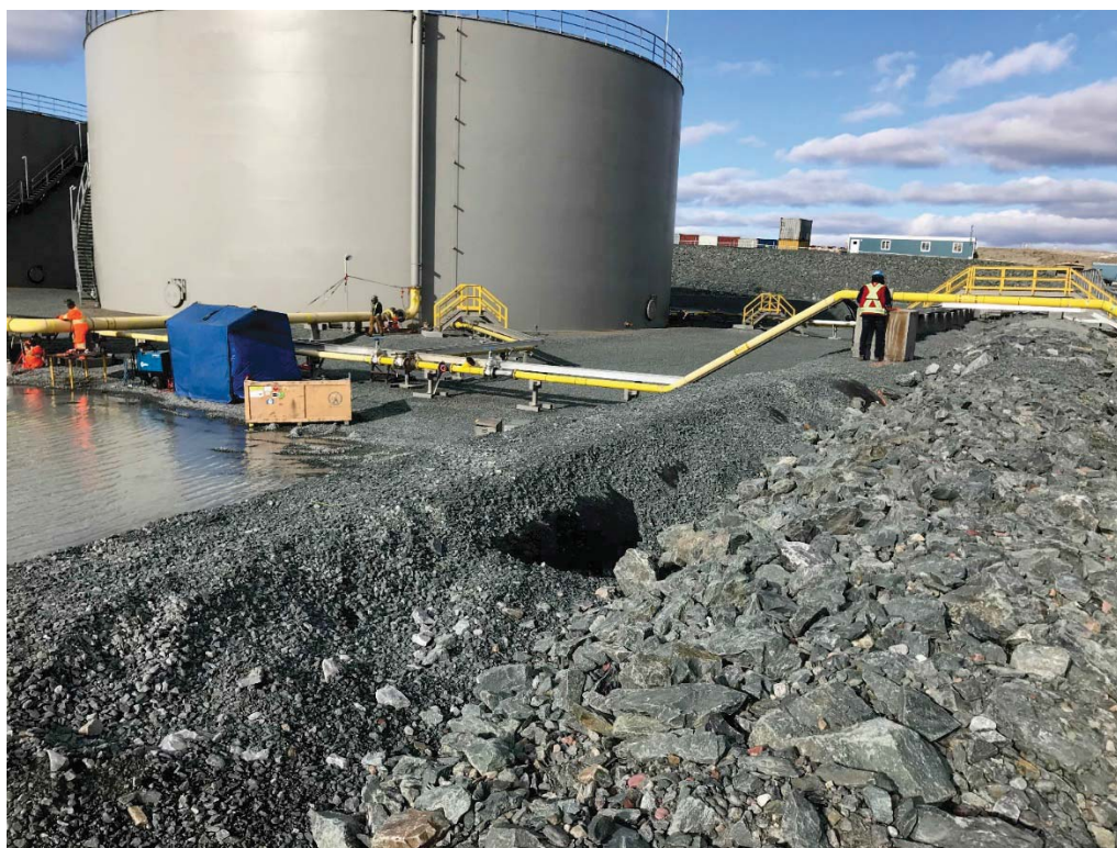
Photograph 10: Itivia Fuel and Laydown Area, Liner Exposed on Crest of East Berm. (14 September 2018).
