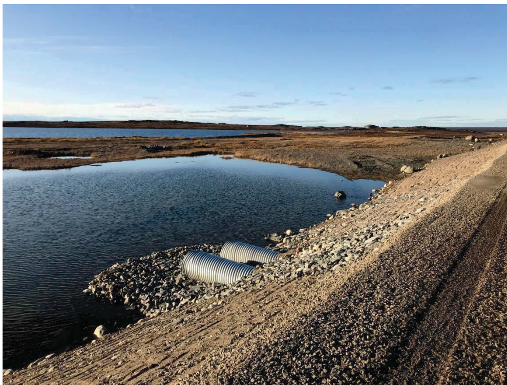
Photograph 48: Culvert 13 Outlets, Ponded Water Observed Downstream Below the Culvert Inverts and Against the Road Embankment Toe, Looking Northwest (14 September 2018)
