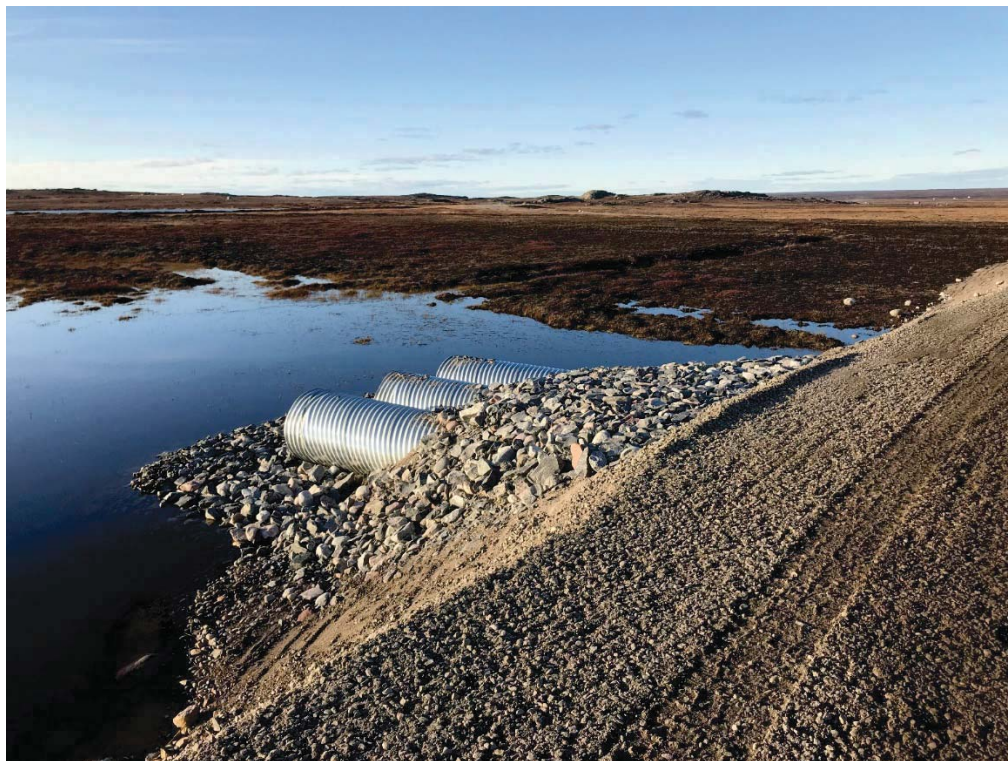
Photograph 50: Culvert 14 Outlets, Ponded Water Below Inverts and Along Road Embankment Toe, Looking Northwest (14 September 2018)
