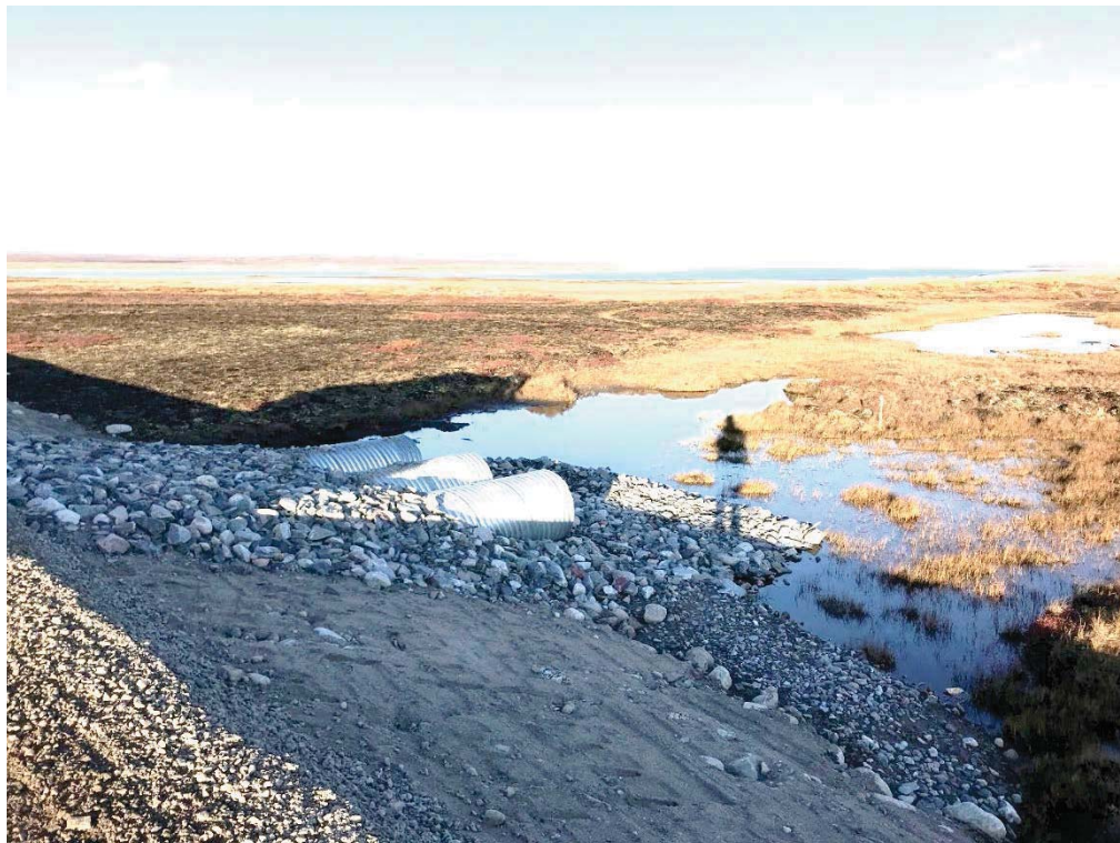
Photograph 49: Culvert 14 Inlets, Ponded Water Upstream and Below Inverts, Looking Northeast (14 September 2018)
