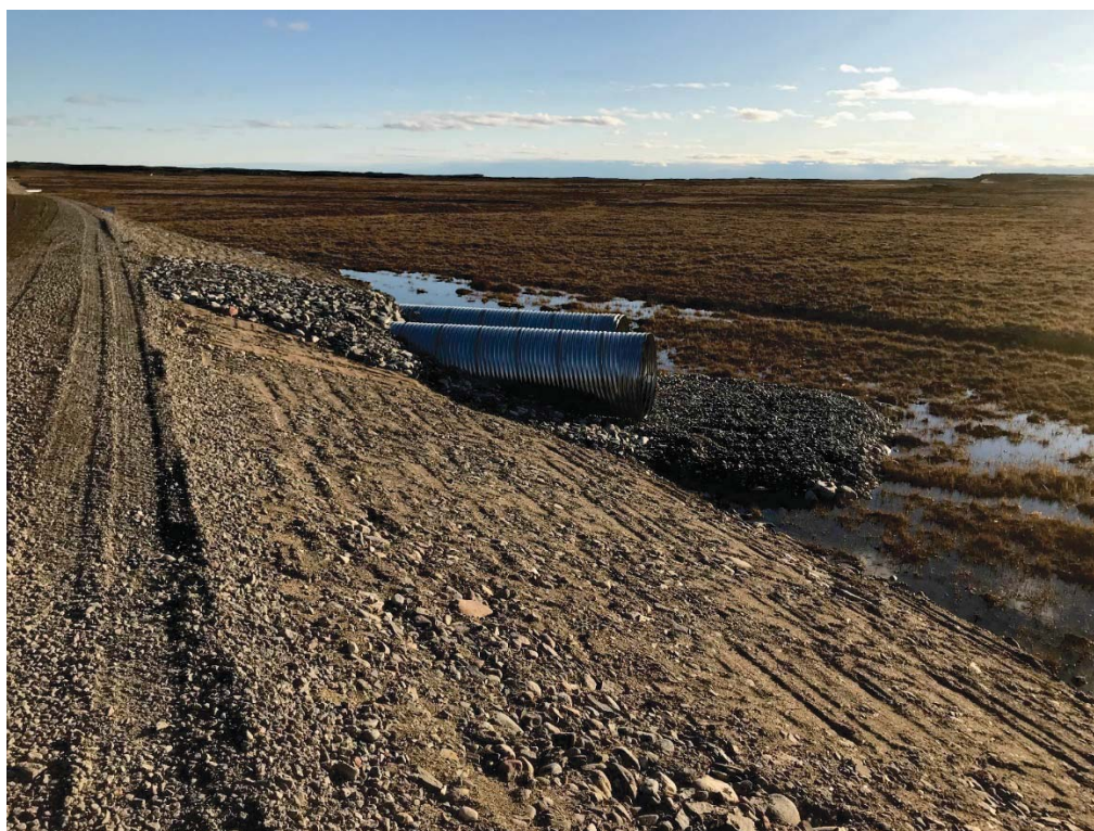
Photograph 46: Culvert 12b Outlets, Ponded Water Below the Inverts and Against Road Embankment Toe, Looking South (14 September 2018)
