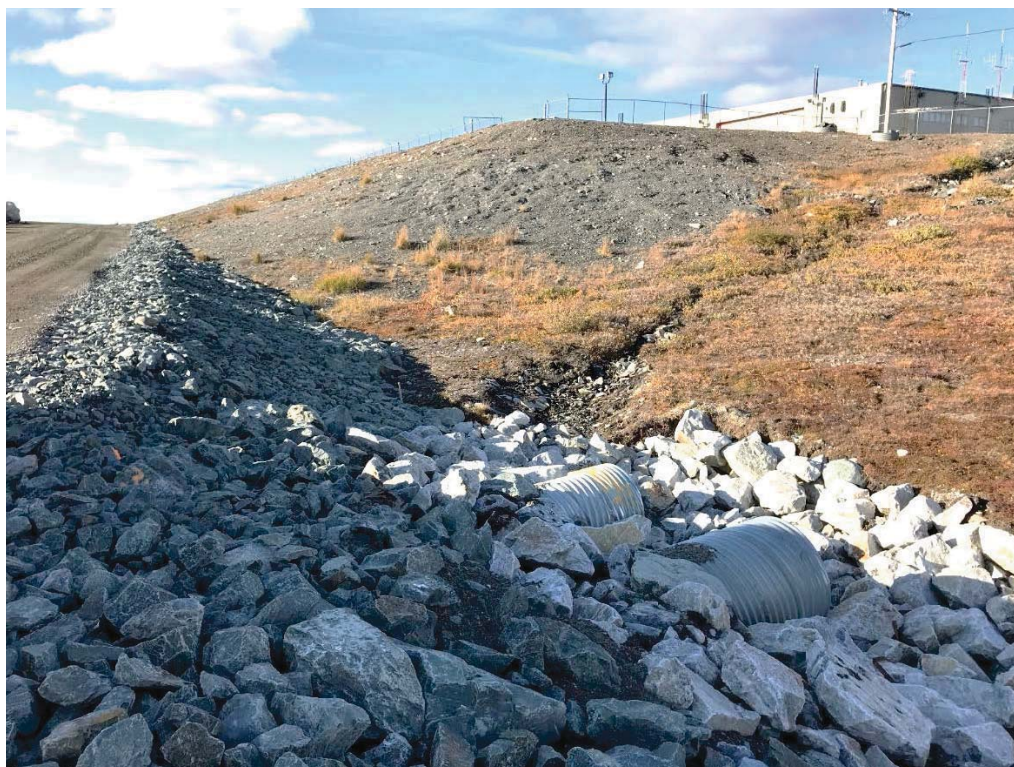
Photograph 14: Inlets for Culvert C03, Looking North. Upstream Channel Erosion (14 September 2018)
