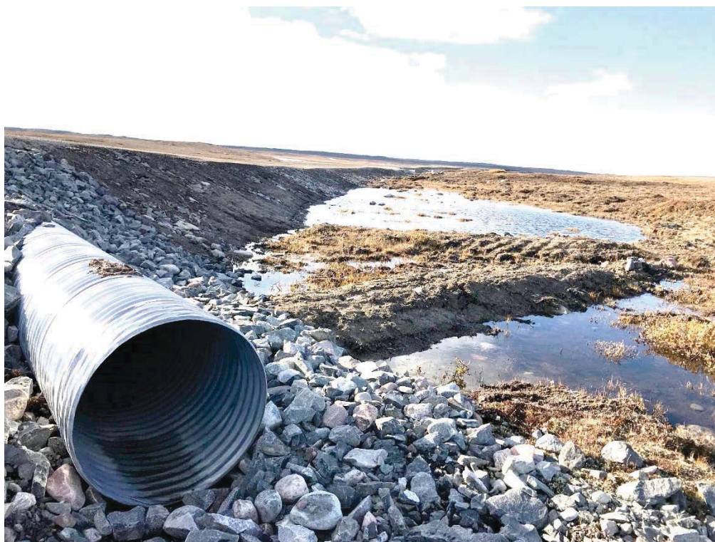
Photograph 22: Diversion Berm West of Culvert C06. Water Ponded Adjacent to Road. Looking Northwest (14 September 2018)
