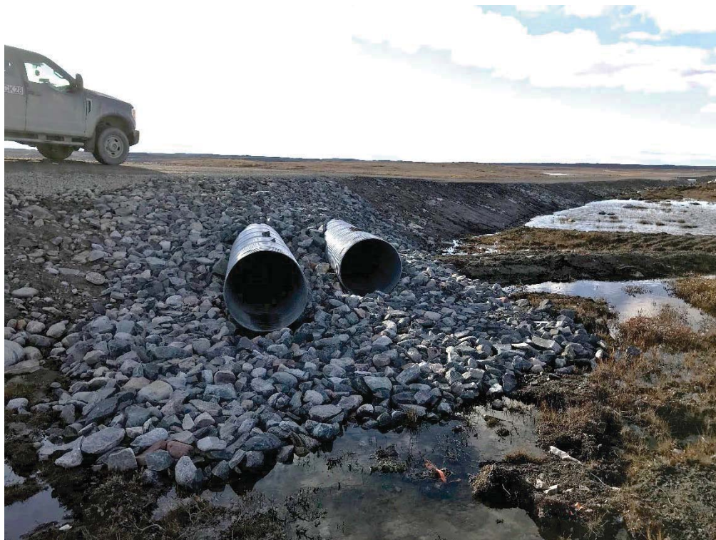
Photograph 21: Inlets for Culvert C06, Looking Northwest. Water Ponded Adjacent to Road Near Inlets (14 September 2018)
