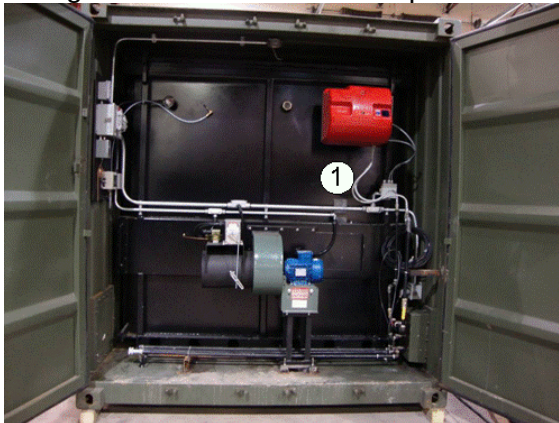
Primary Chamber Burner Flexible lines
