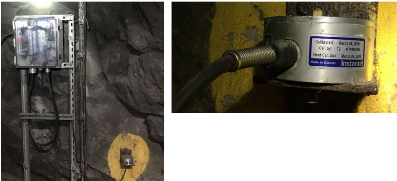
Figure 3-3 Underground Installation (L75)
