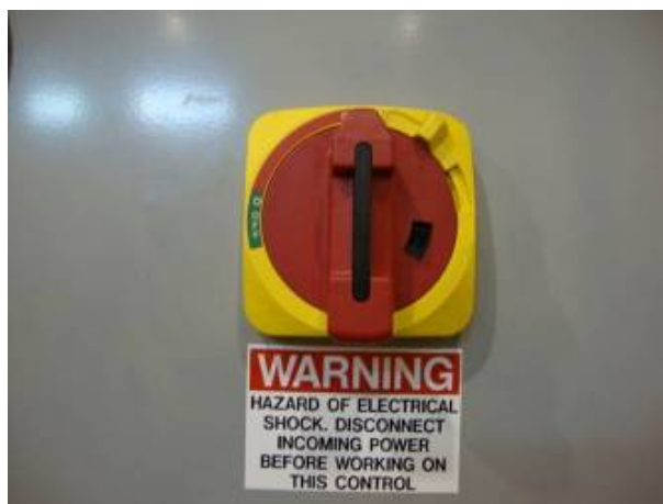
Power is ON in this position
