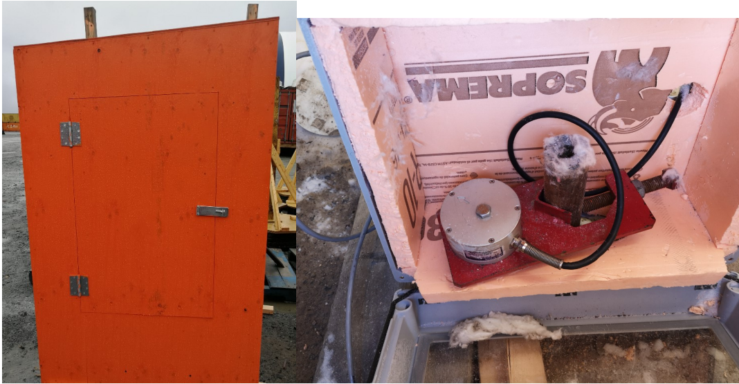
Figure 6. Surface Installation (Shelter & installation inside)
