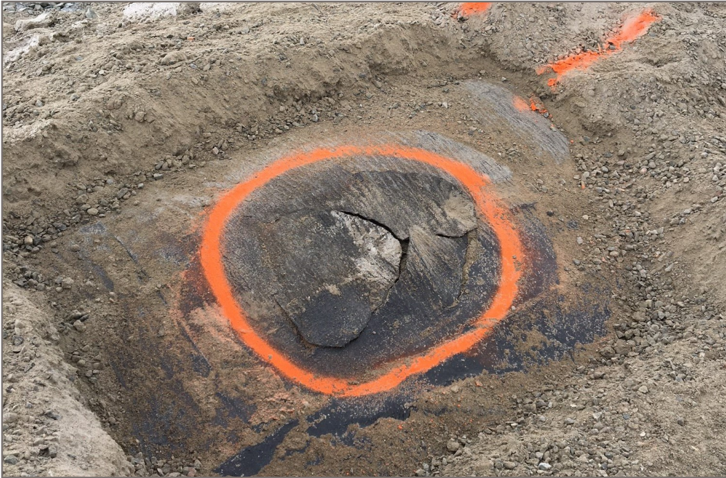
Photo 50: Top Liner punctured by excavator while placing Type C material; Station 1+040
