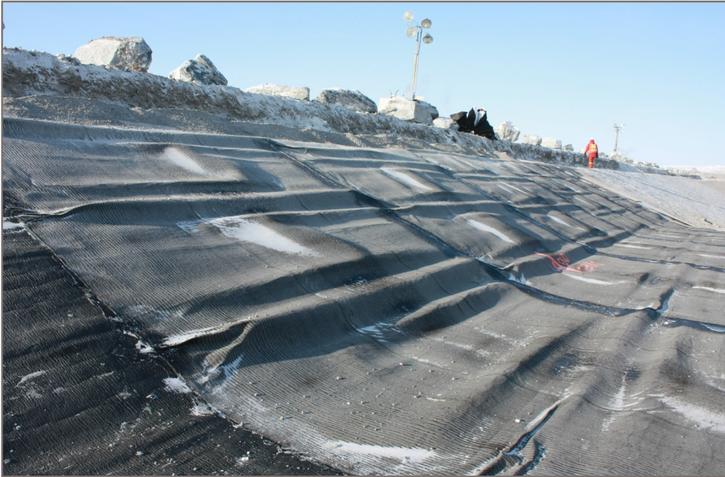
Photo 54: Excessive wrinkling on Liner Panels 62 to 66
