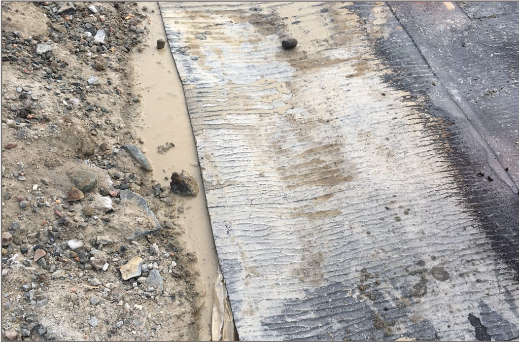
Photo 56 Water ponding at under liner hinge point View at Station 1+390
