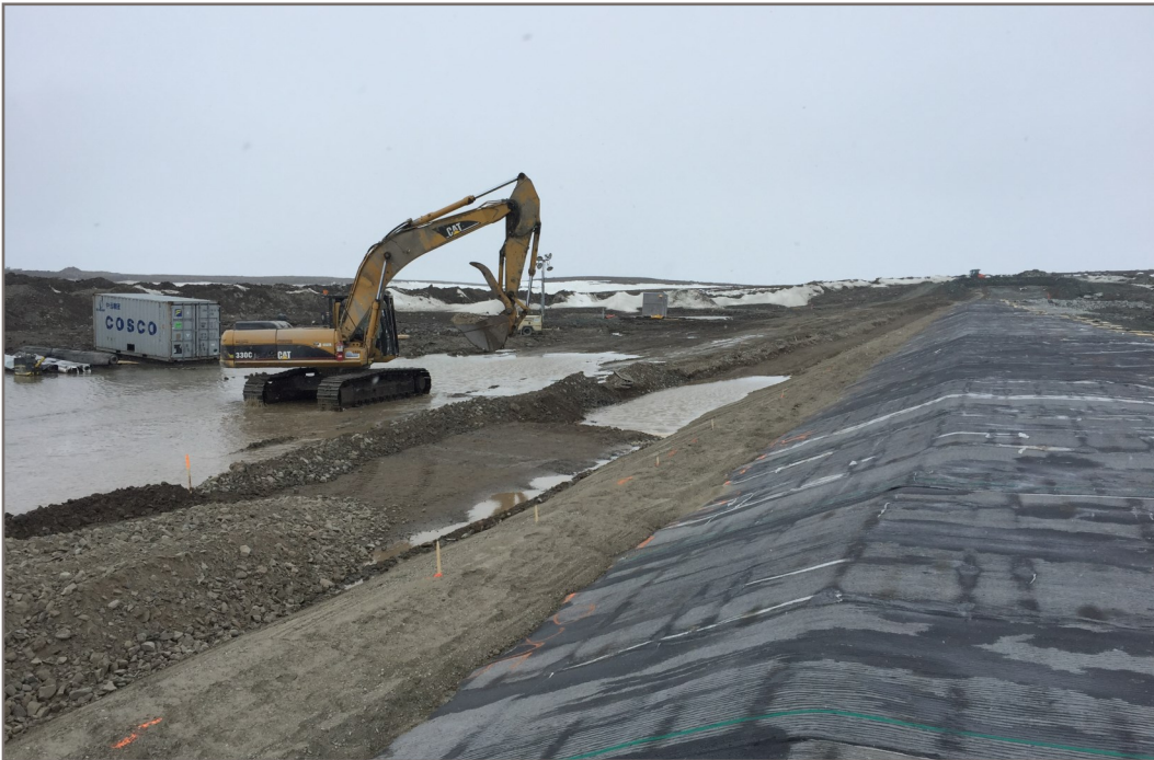
Photo 57: Water breach over Type H upstream material on working platform View from Station 1+400 facing down chainage
