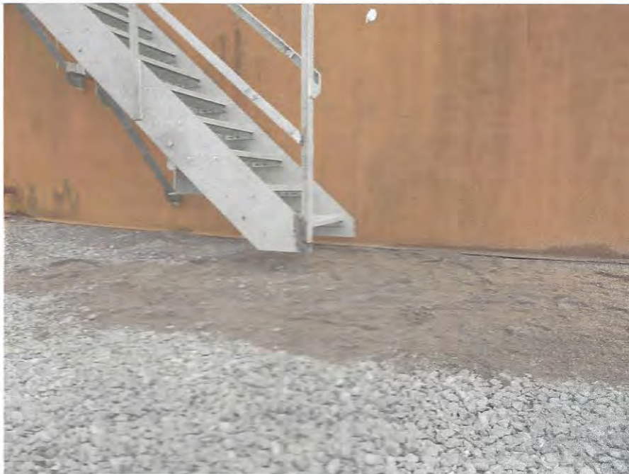
Photo of stairway after bottom step removed
