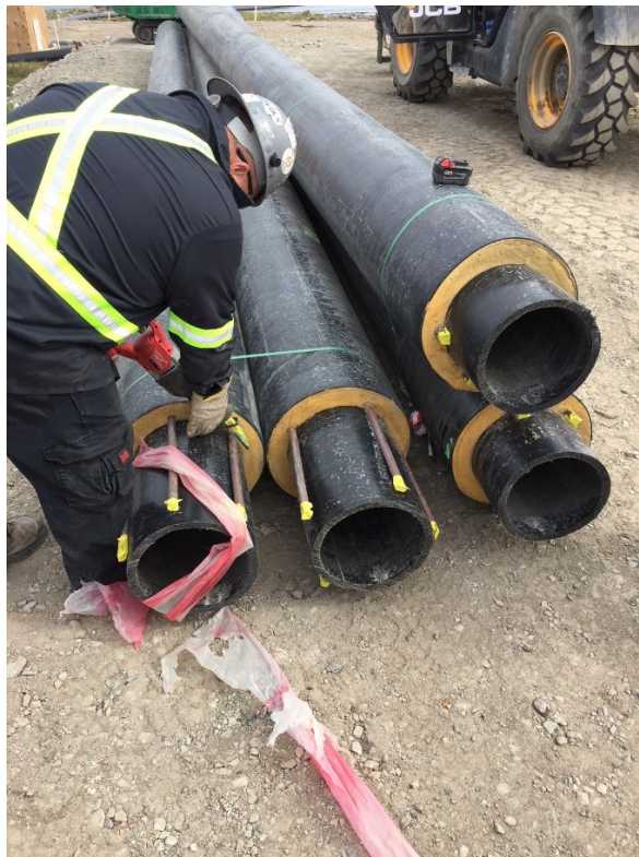
Photo 4 Meliadine's fresh water intake insulated and heat traced piping
