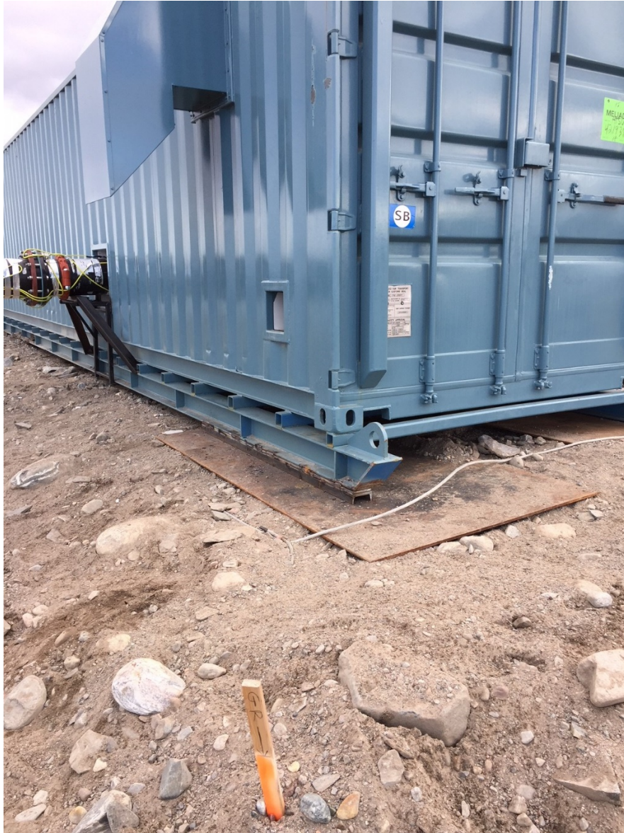
Photo 5 Meliadine Fresh Water Pumping Station
