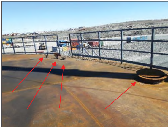
Nozzles 3 to 6 of 13 on top tank
