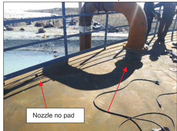
Nozzles 10, 11 of 13 on top tank
