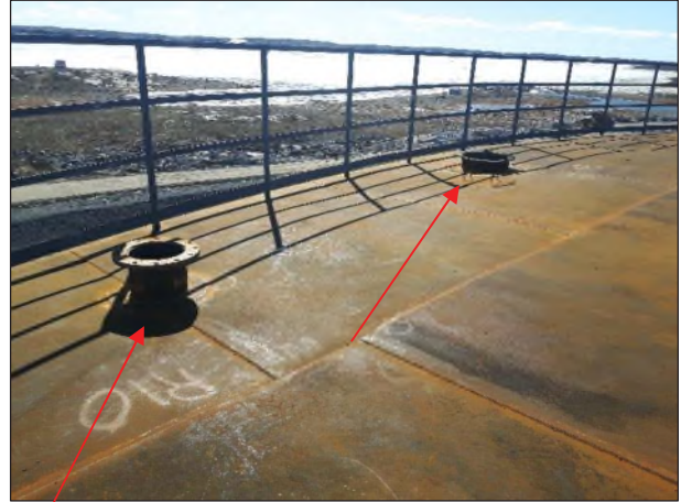
Nozzles 1, 2, of 13 on top tank
