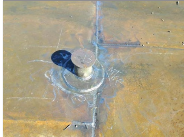
Nozzles 13 of 13 on top tank
