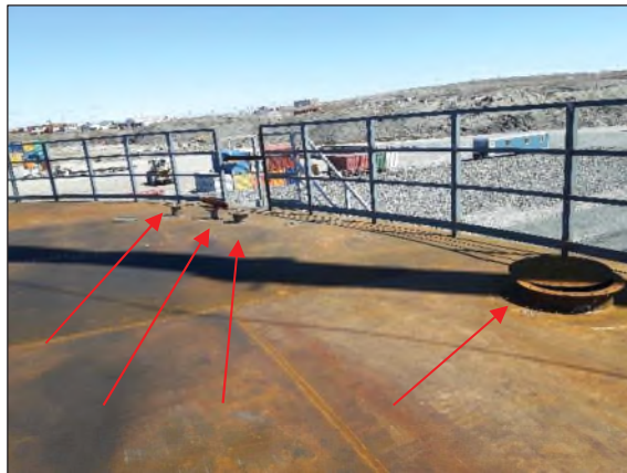
Nozzles 3 to 6 of 13 on top tank
