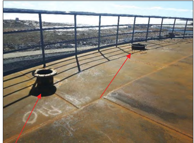
Nozzles 1, 2, of 13 on top tank
