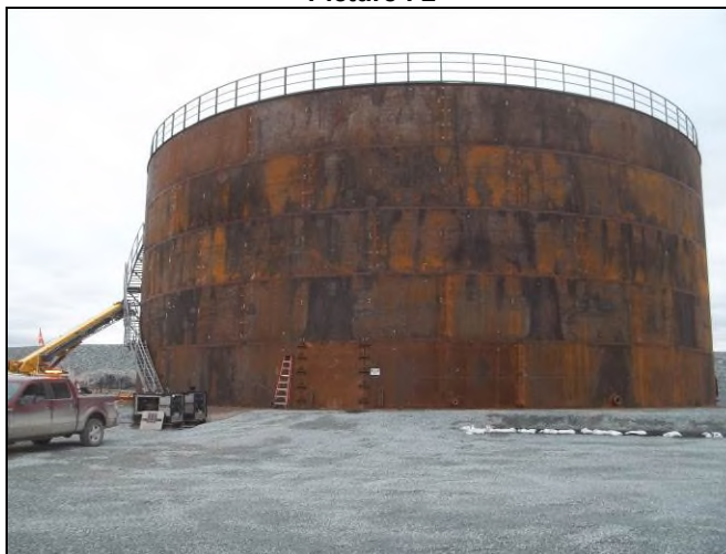
View of tank 2
