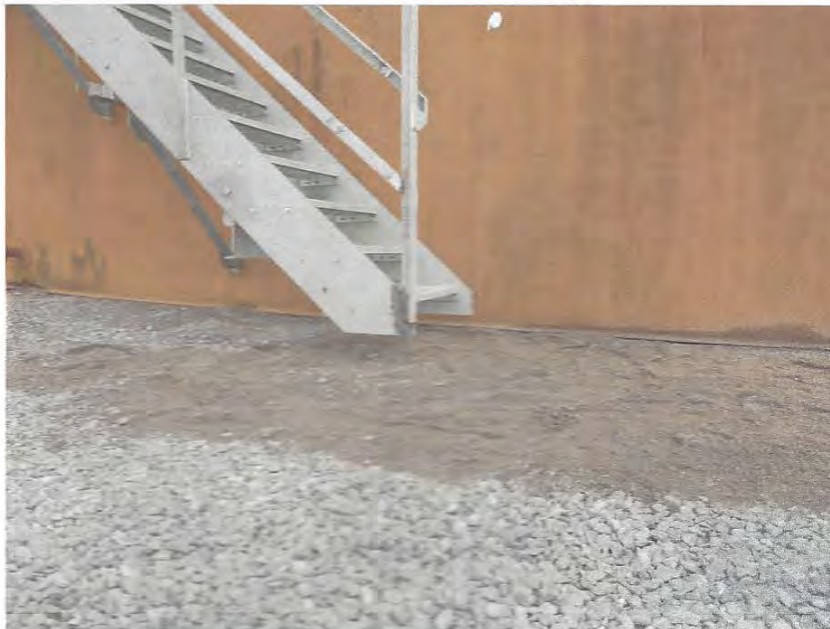
Photo of stairway after bottom step removed
