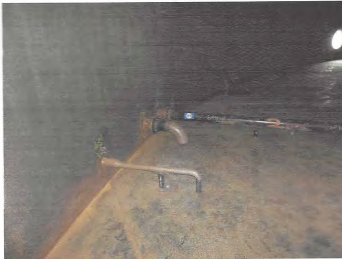
Photo of Water Draw Off Valve with 6" Extension
