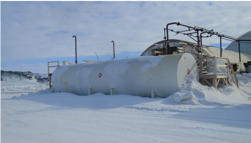
Photo 4 Construction Genset Horizontal Fuel Storage Tanks (looking south-east)
