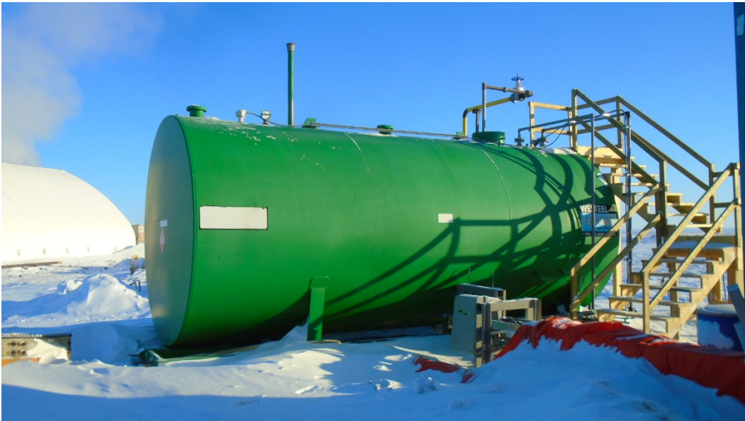
Photo 2 Mine Ventilation and Heating System Horizontal Fuel Storage Tank (looking towards Portal 1 and Mine Site Fuel Farm (south-east))
