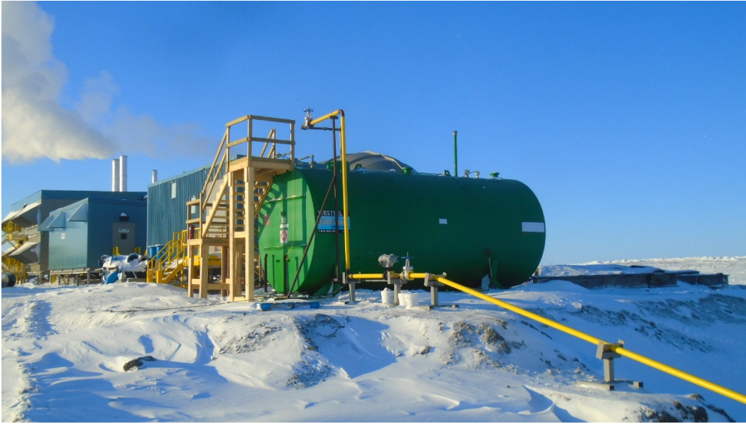
Photo 1 Mine Ventilation and Heating System Horizontal Fuel Storage Tank (looking towards the ventilation system (north-west); yellow pipeline connects the Mine Site Fuel Farm to the horizontal tank)
