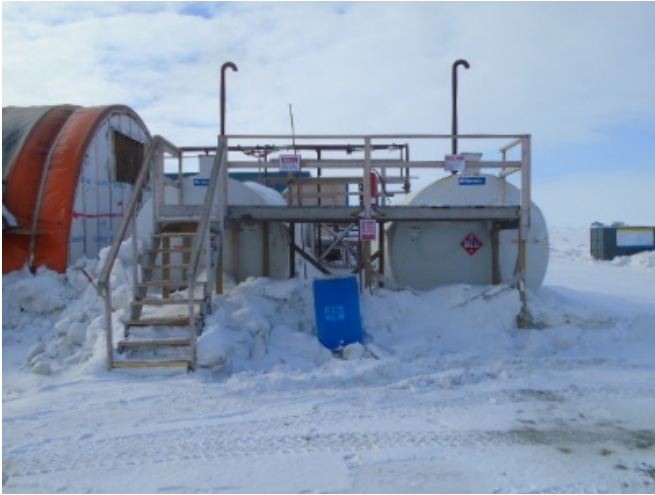
Photo 3 Construction Genset Horizontal Fuel Storage Tanks (looking west)
