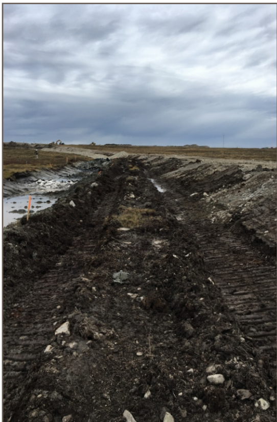
Photo 6: 08 29 2018 Channel3 - Poor bank conditions, ice, and bedrock; Station 1+320 facing up-chainage
