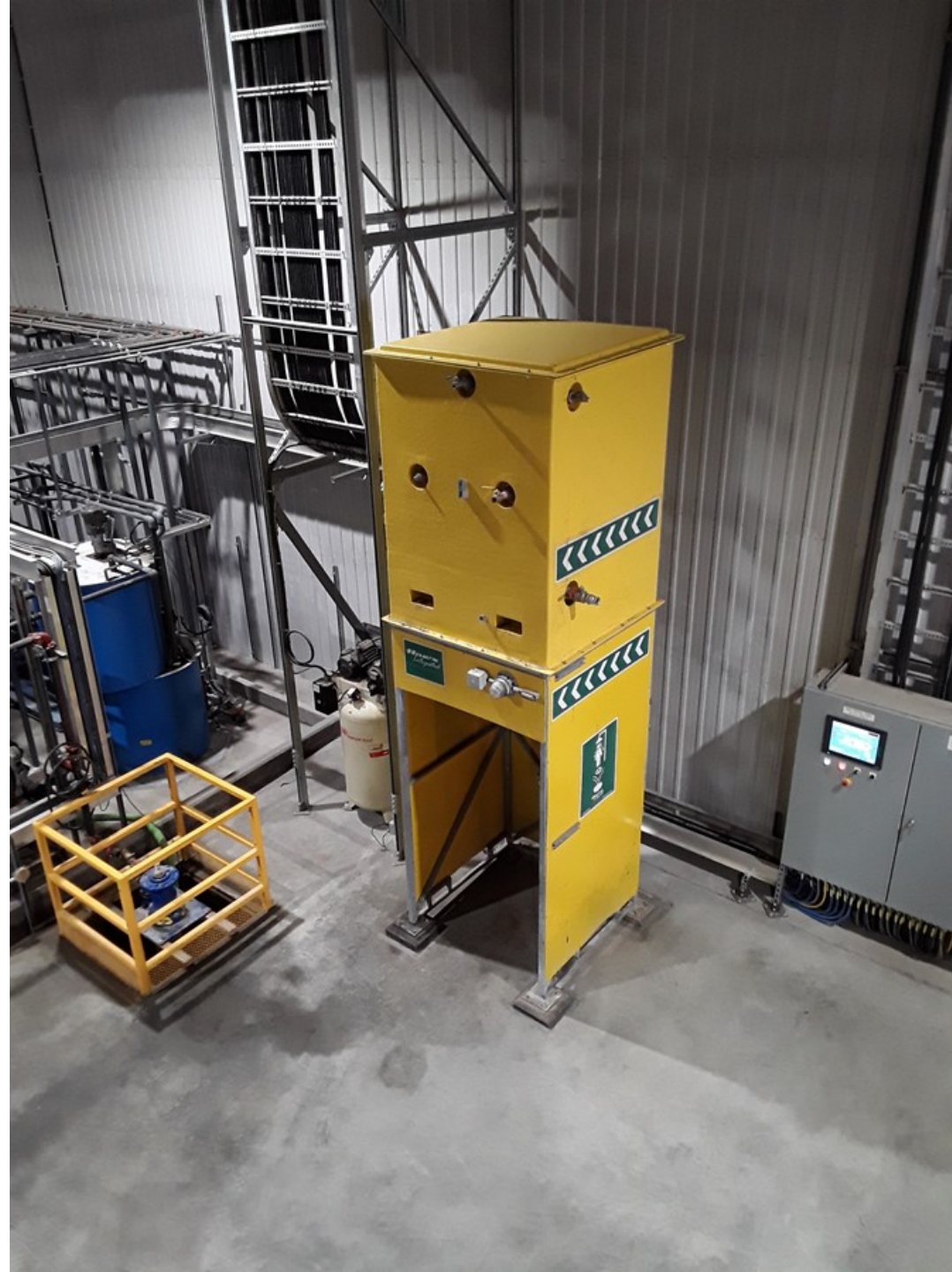
Safety Shower, sump, compressor, HMI
