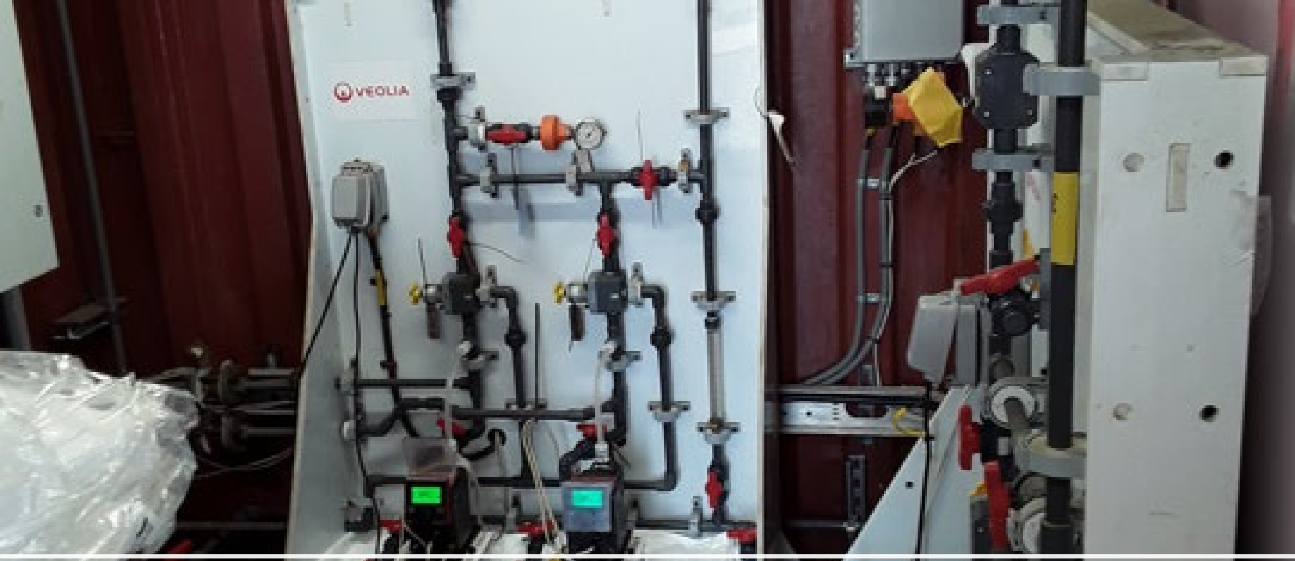
Coagulant dosing Skids
