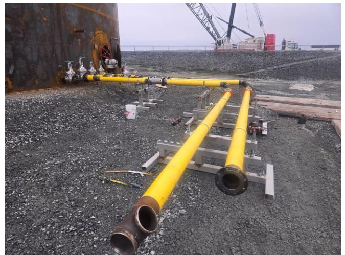
Picture 4 116 – Fuel Tank Farm (Line 116-150-PDI-CC10-0026)
