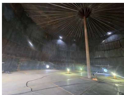
Picture 2 Rankin Inlet Tank#3 (9ML) inside
