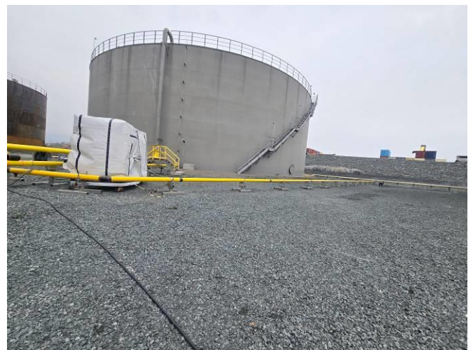
Picture 6 116 – Fuel Tank Farm Line 116-150-PDI-CC10-0115
