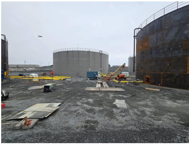
Picture 1 Pipes 116 – Fuel Tank Farm (General view)
