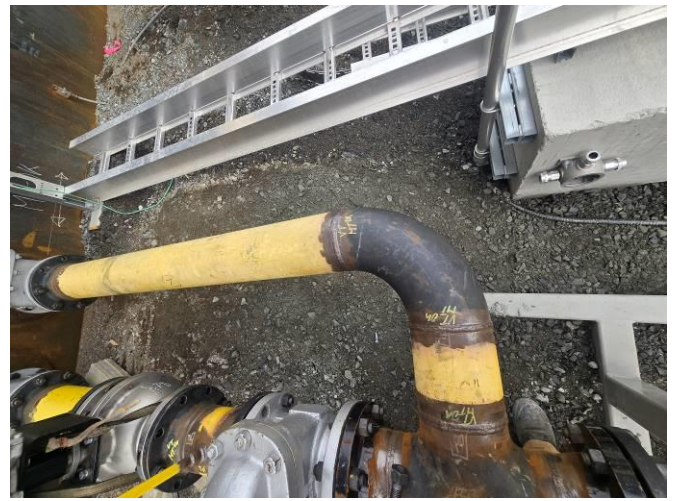
Picture 2 Pipes 116 – Fuel Tank Farm (Line 116-150-PDI-CC10-0111)
