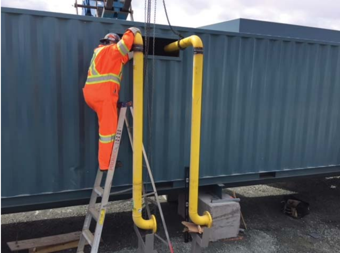
Photo 8 Pipe connexion at Industrial Site Fuel Farm pumping station
