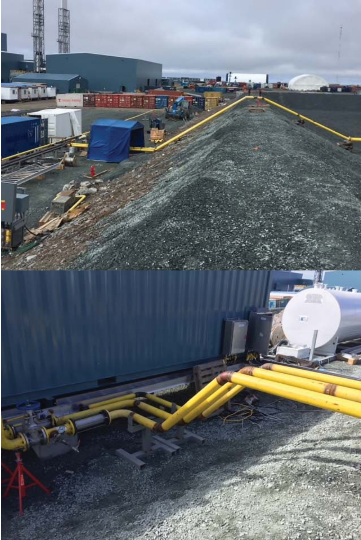
Photos 21 and 22 Piping arrangement between Industrial Site Fuel Farm tanks, pumping station and Power Plant
