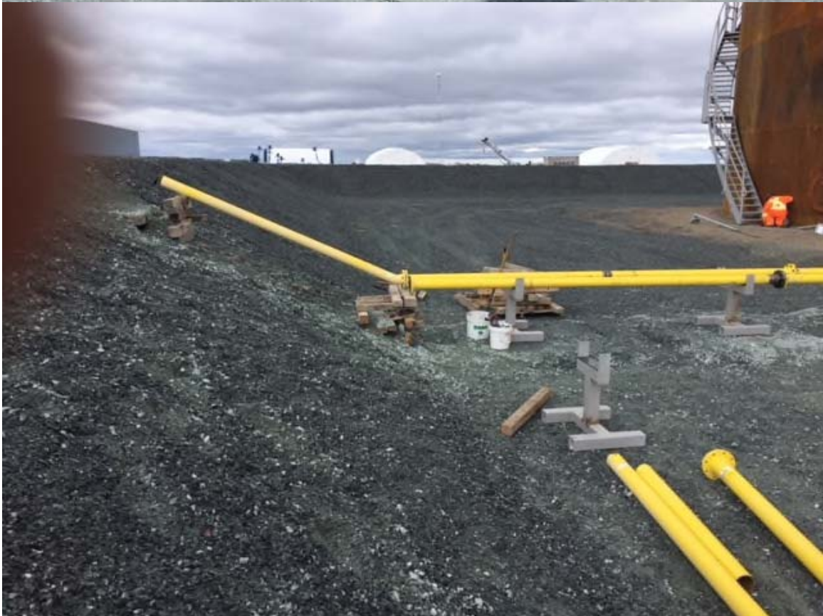
Photo 14 Piping within Industrial Site Fuel Farm
