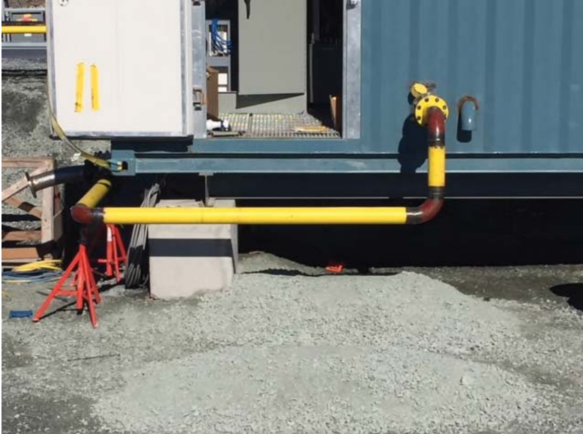
Photos 19 and 20 Piping arrangement between Industrial Site Fuel Farm tanks, pumping station and Power Plant
