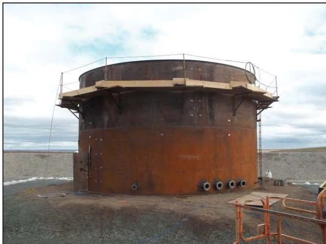
View of tank # 5
