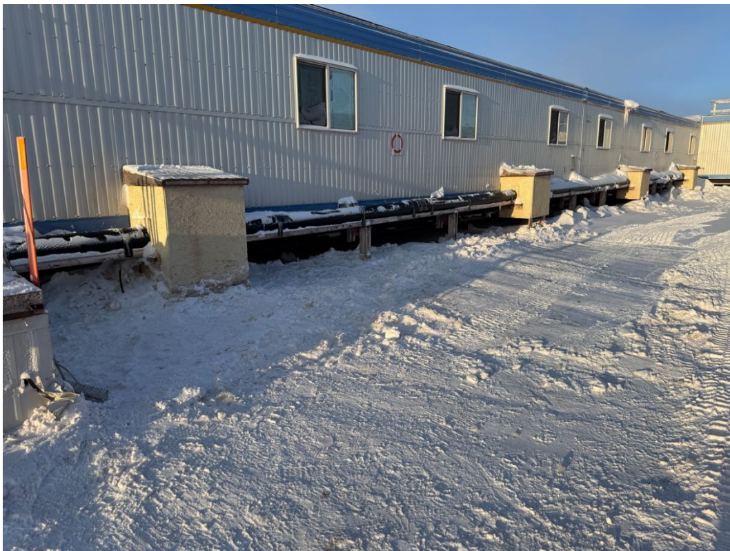
Photo 4: Near Final Clean-Up of Spill #2026-062 at the Milne Port PSC – April 18, 2026
