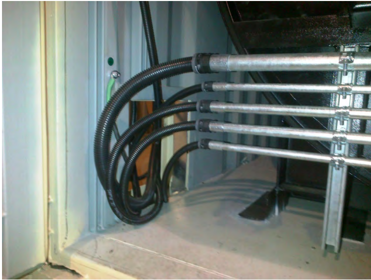
Flexible conduit in Container 2 (secondary chamber)
