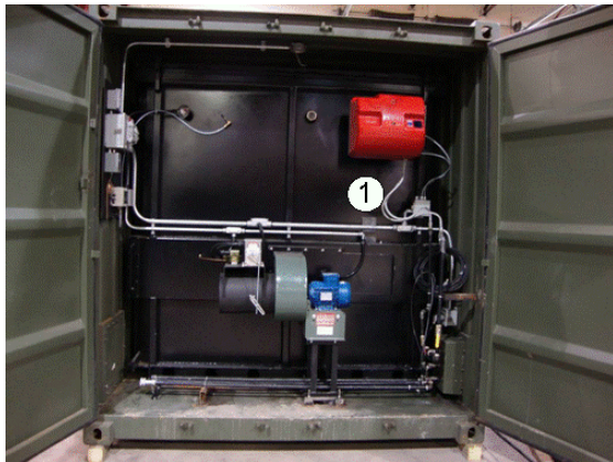
Primary Chamber Burner Flexible lines (1 Above)
