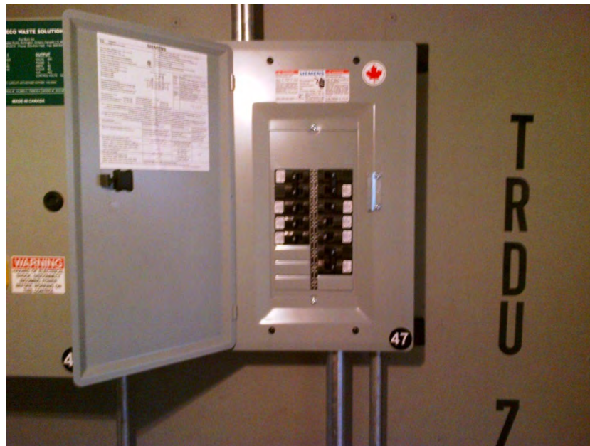
Switch on all incinerator breakers in the Breaker Panel
