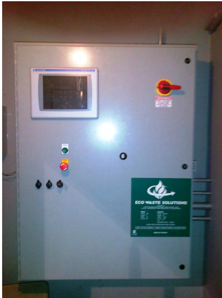
Front View: Main Control Panel
