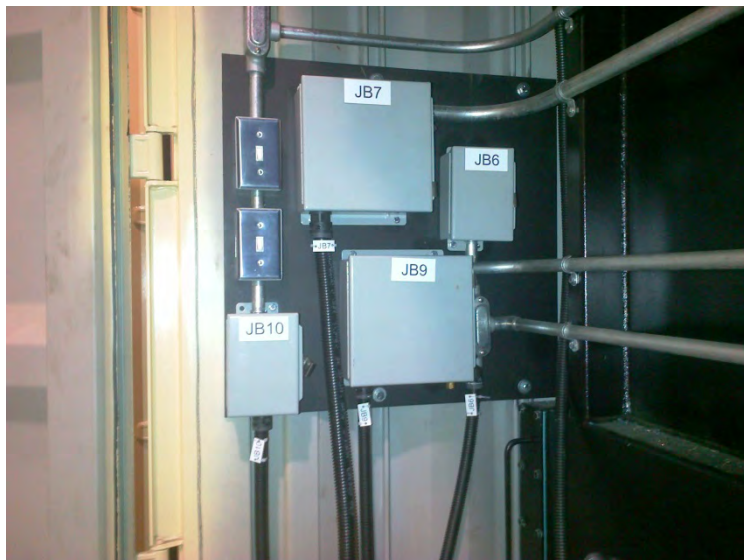
Junction Boxes in container 1 (primary chamber)
