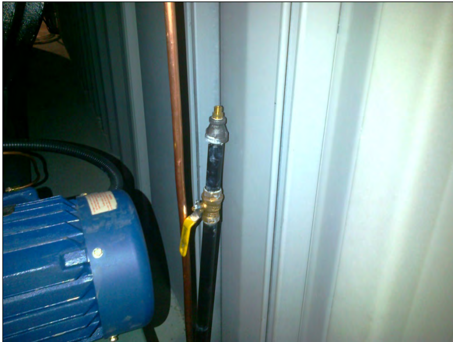
Compressed air quick connect for Waste Oil Burner
