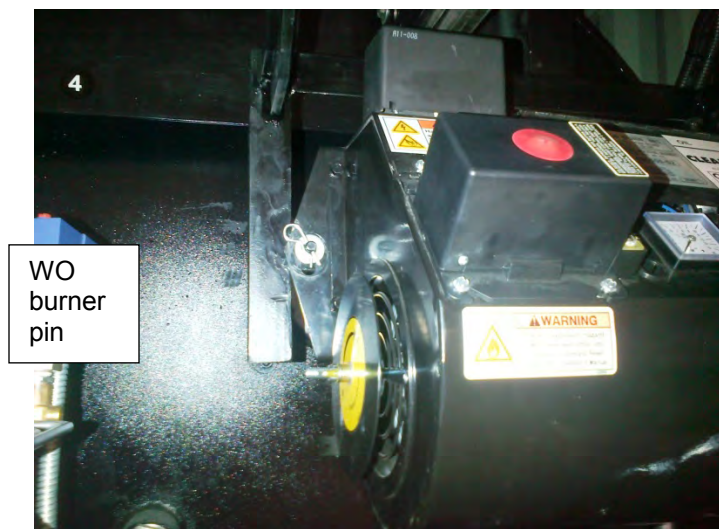
Waste oil burner secured with pin
