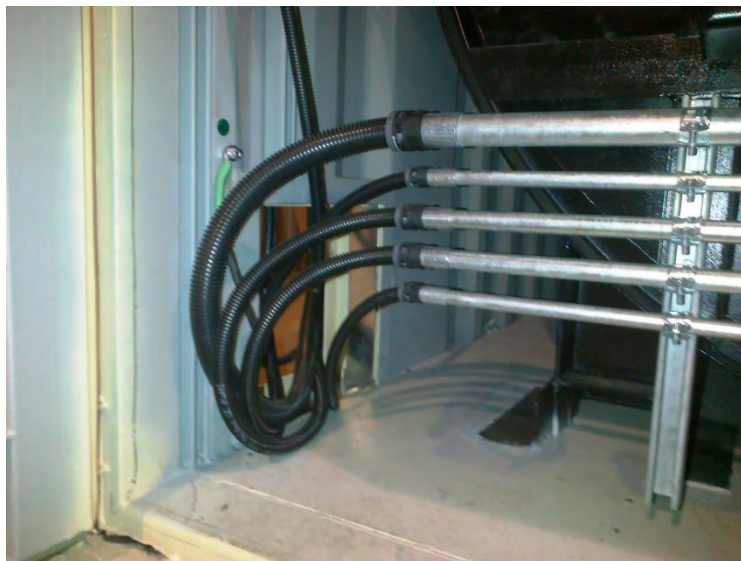
Flexible conduit in Container 2 (secondary chamber)
