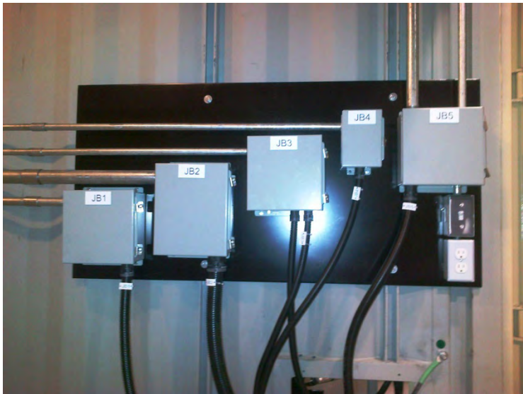
Junction Boxes in container 3 (control container)
