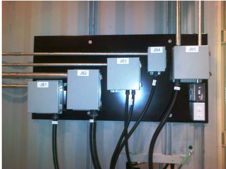
Junction Boxes in container 3 (control container)
