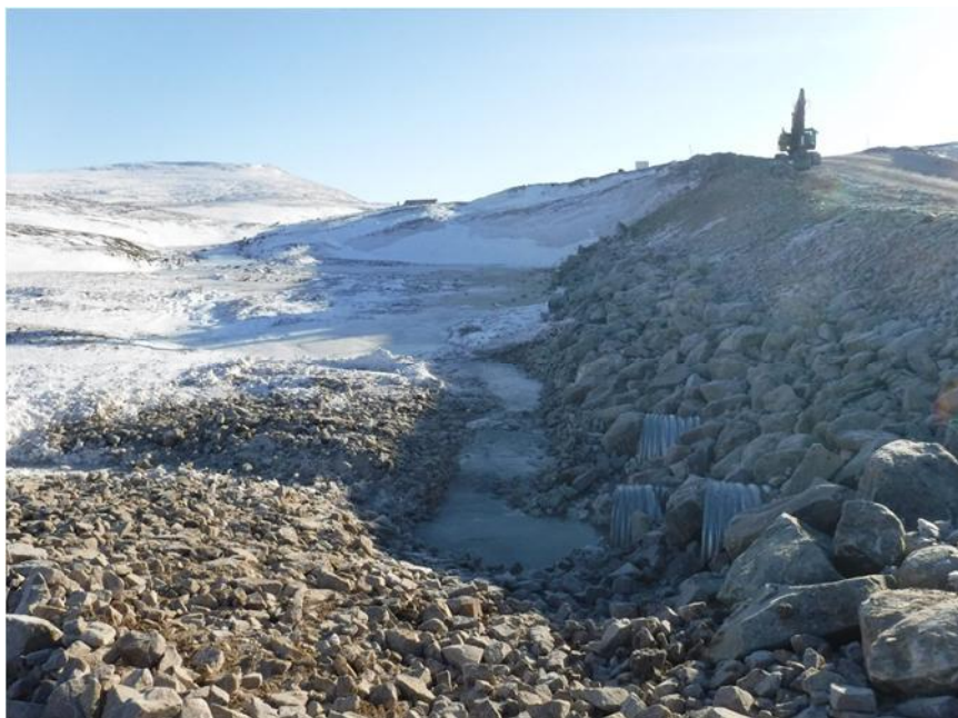
Figure 3. BG01 US installed 17-10-09
