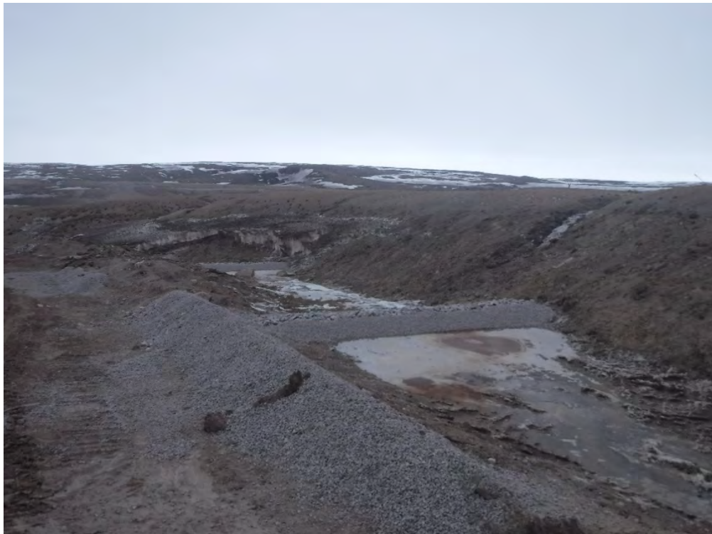
May 22, 2018: Check Dams in Camp Lake Settling Pond Drainage Channel After Construction Upgrades
