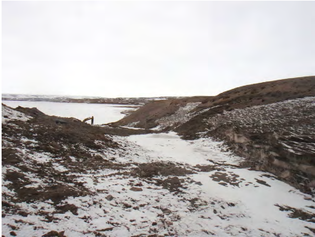
May 20, 2018: Check Dams in Camp Lake Settling Pond Drainage Channel Before Construction Upgrades
