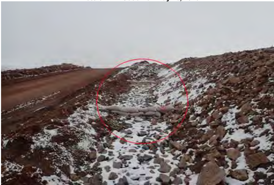
Photo 4: BG-01 Downstream Ditch with Sand Bags (May 18, 2020)
