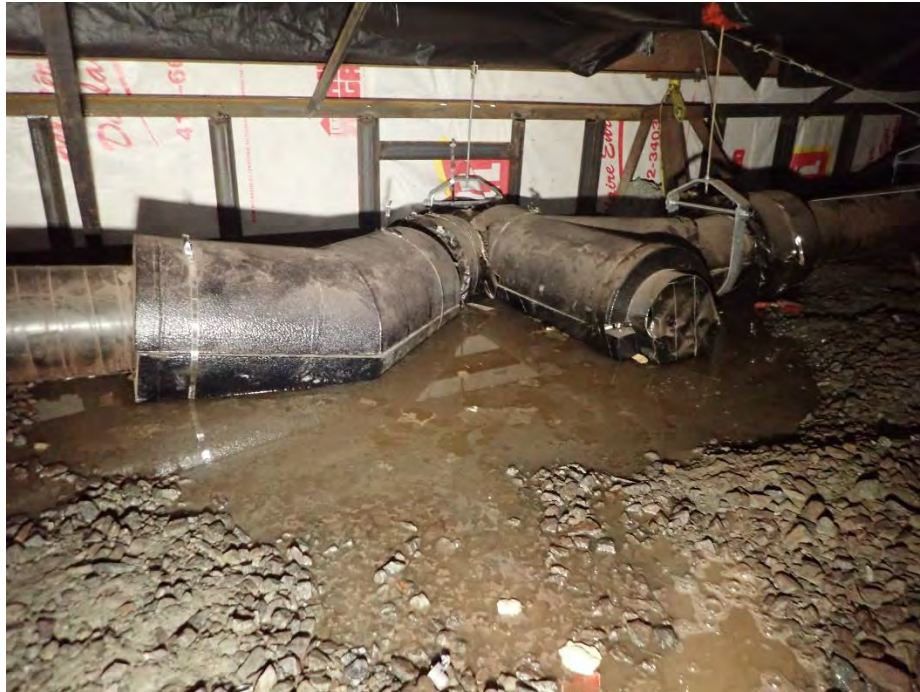
Photo 1. Spill location before clean-up
