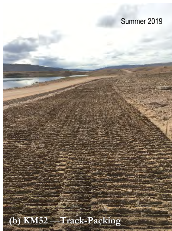
Photo 10. KM52 — Rough and loose (a) and track-packing (b).
