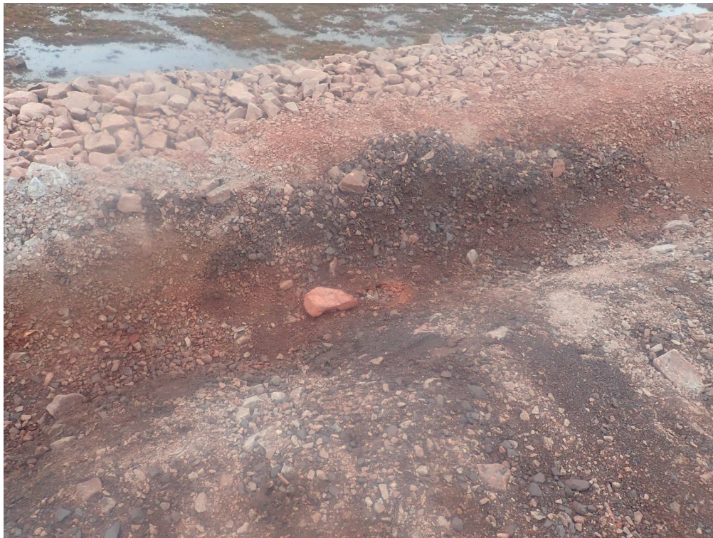
Photo 2. Seepage Location within West Ore Pad Ditch (July 2, 2021)
