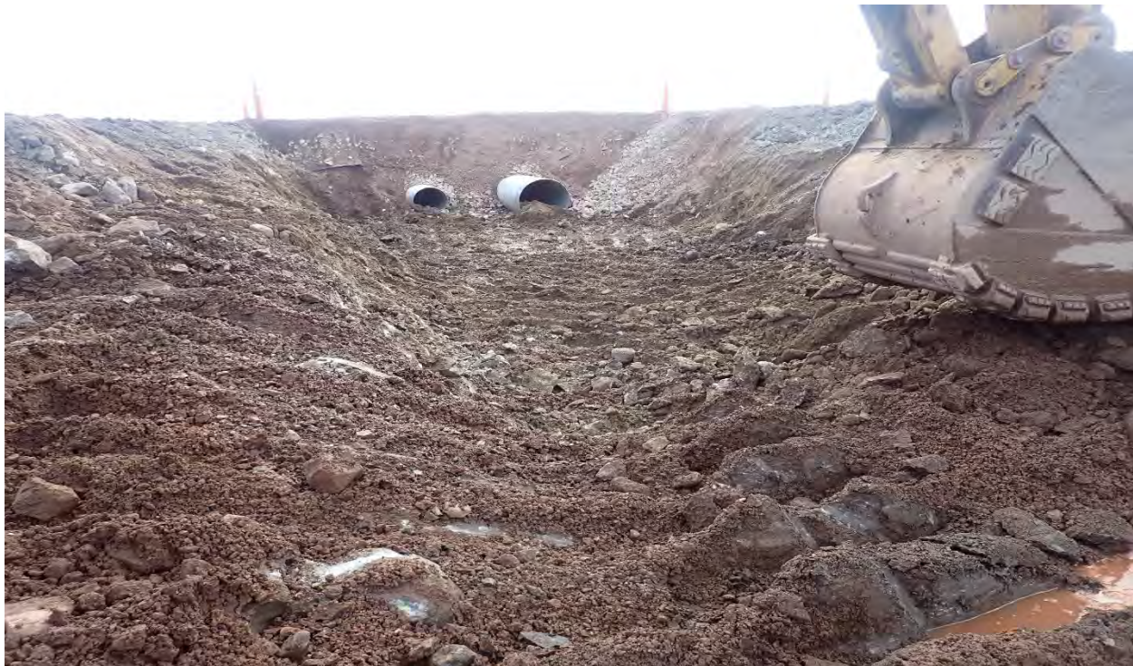
Photo 10. Downstream looking south, crossing excavated to road centreline and existing culverts removed, new upstream culvert visible, 2025-06-23
