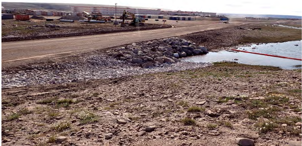
Photo 12. Downstream embankment armoured with over-sized rip rap, rock check dams reconstructed in roadside swale, 2025-06-28
