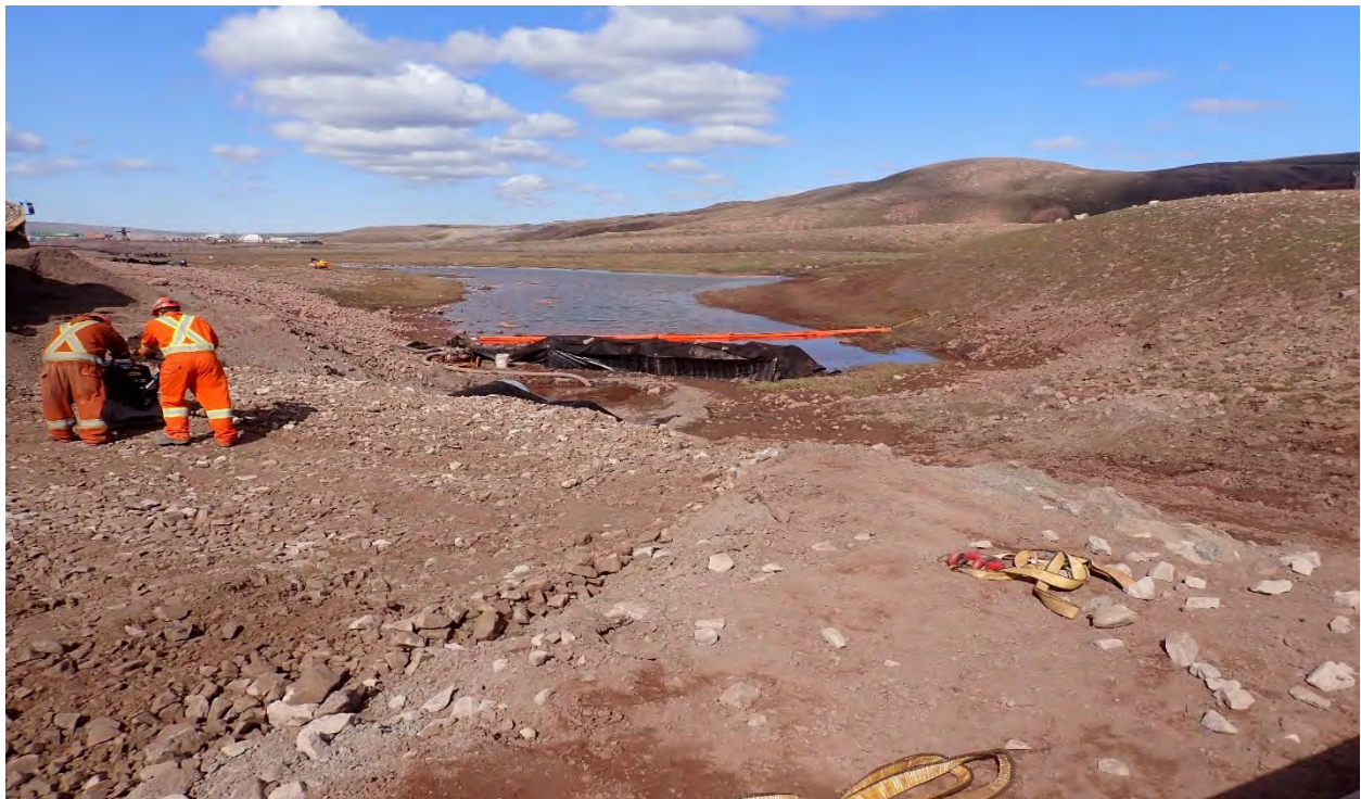
Photo 12. Downstream looking north, road base compaction, watercourse isolation and downstream silt curtain, 2025-06-24
