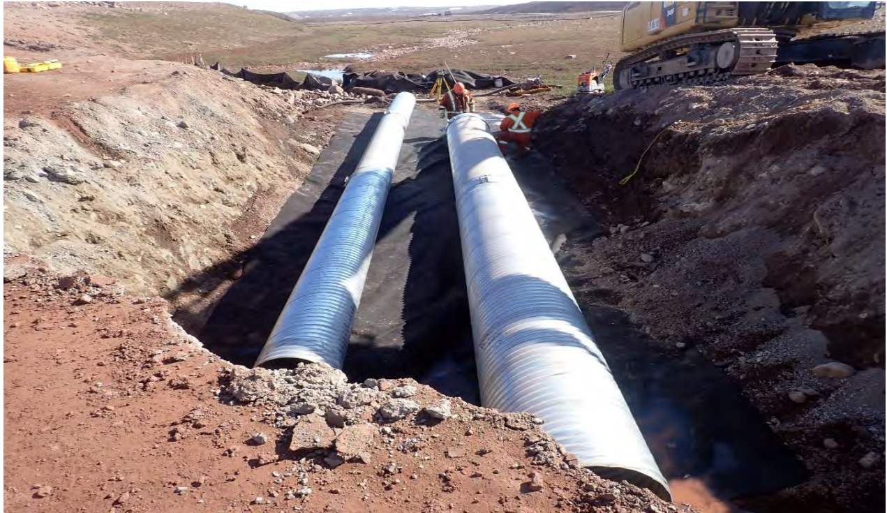
Photo 7. High flow and low flow culverts installed in the upstream half of the crossing, 2025-06-22
