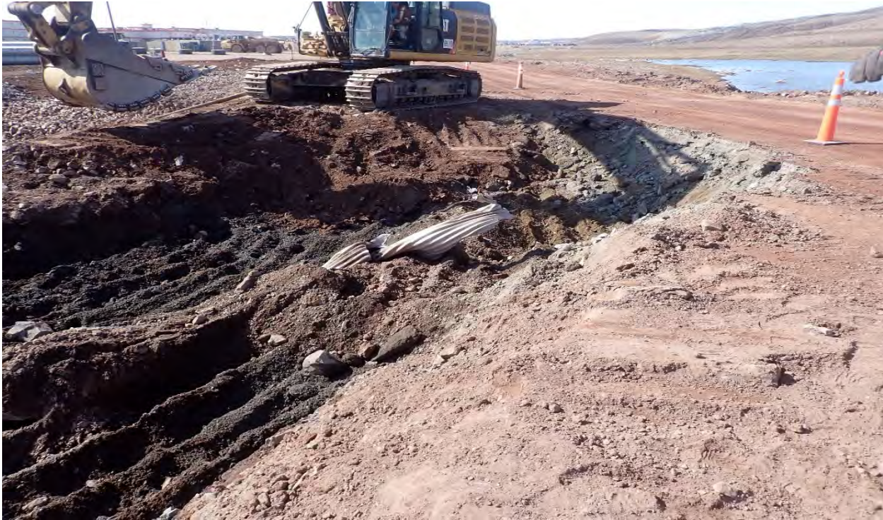
Photo 3. Excavating and removing existing upstream culverts, up to the road centre line, 2025-06-21
