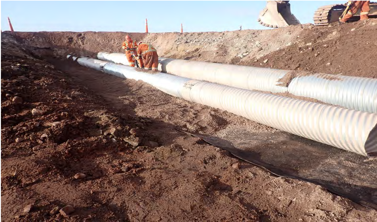
Photo 11. Downstream looking south west, connection of downstream culvert section to upstream section, assembly of culverts, 2025-06-24
