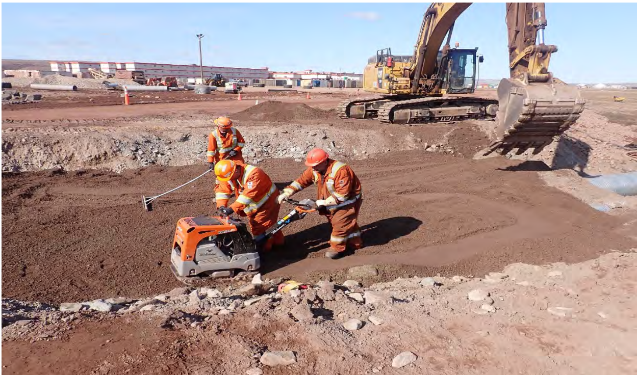
Photo 12. Downstream looking north west, compaction of \frac{3}{4} " minus around and on top of culverts, 2025-06-24
