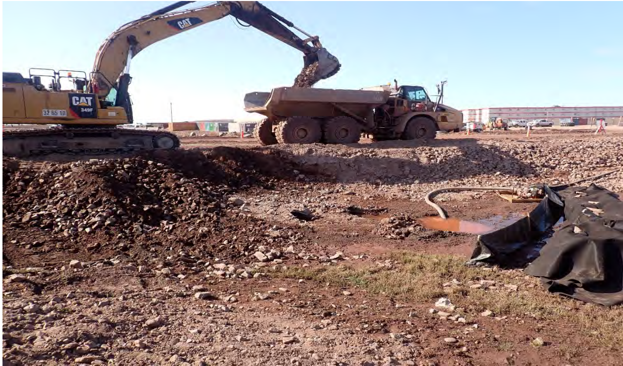
Photo 9. Downstream looking south west, de-watering work area, removing existing rip rap embankment, 2025-06-23
