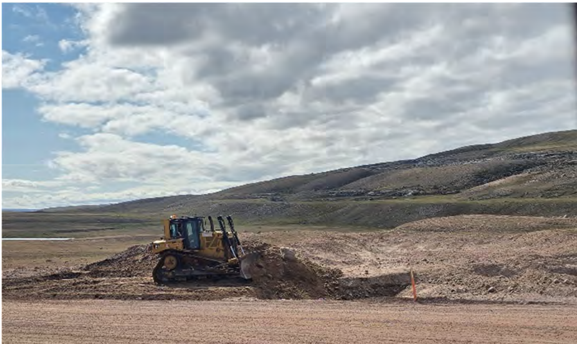
Figure D2. Regrading of Borrow Pit 71 using a CAT D6 dozer, July 2025
