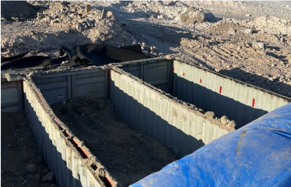
Photo 5. Abutment anchors partially filled
