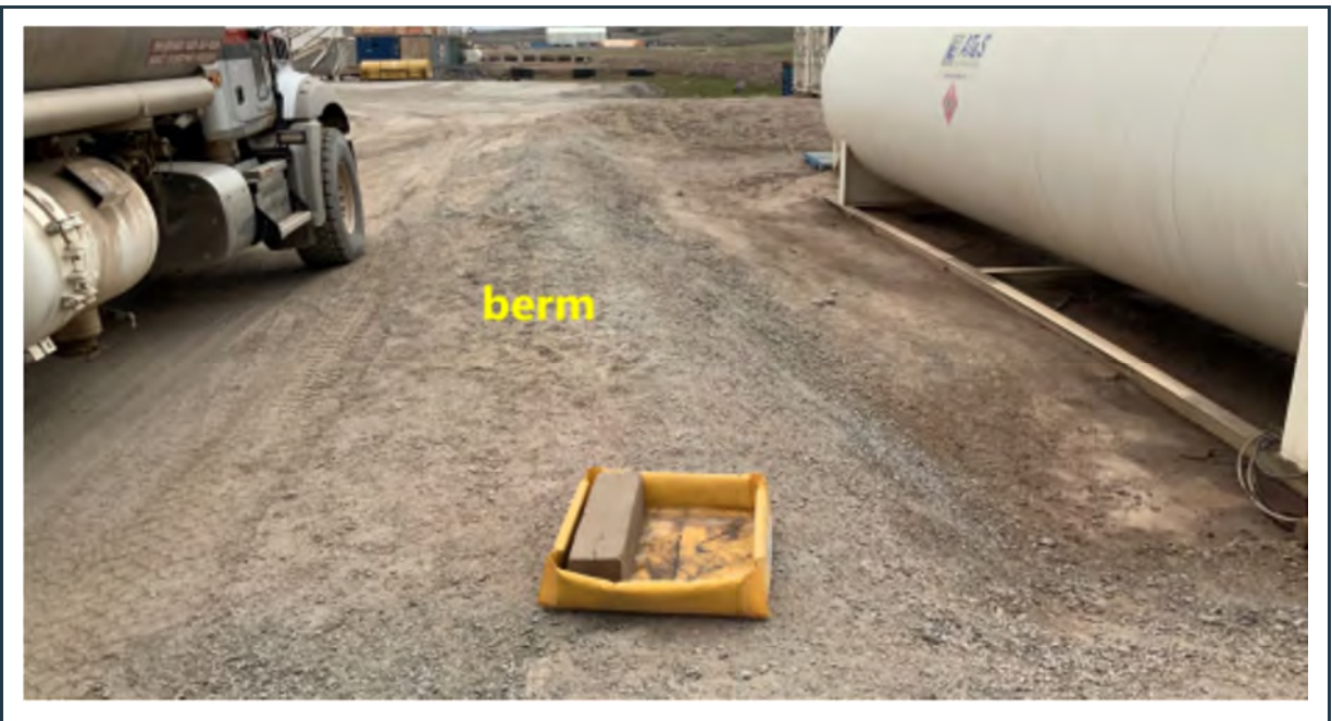
Figure 39: View of the well-maintained sand and gravel berm at the lined jet-fuel storage facility.
