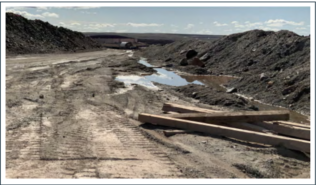
Figure 45: Drainage problems still exist at the first quarry level. Surface drainage shall be rectified.
