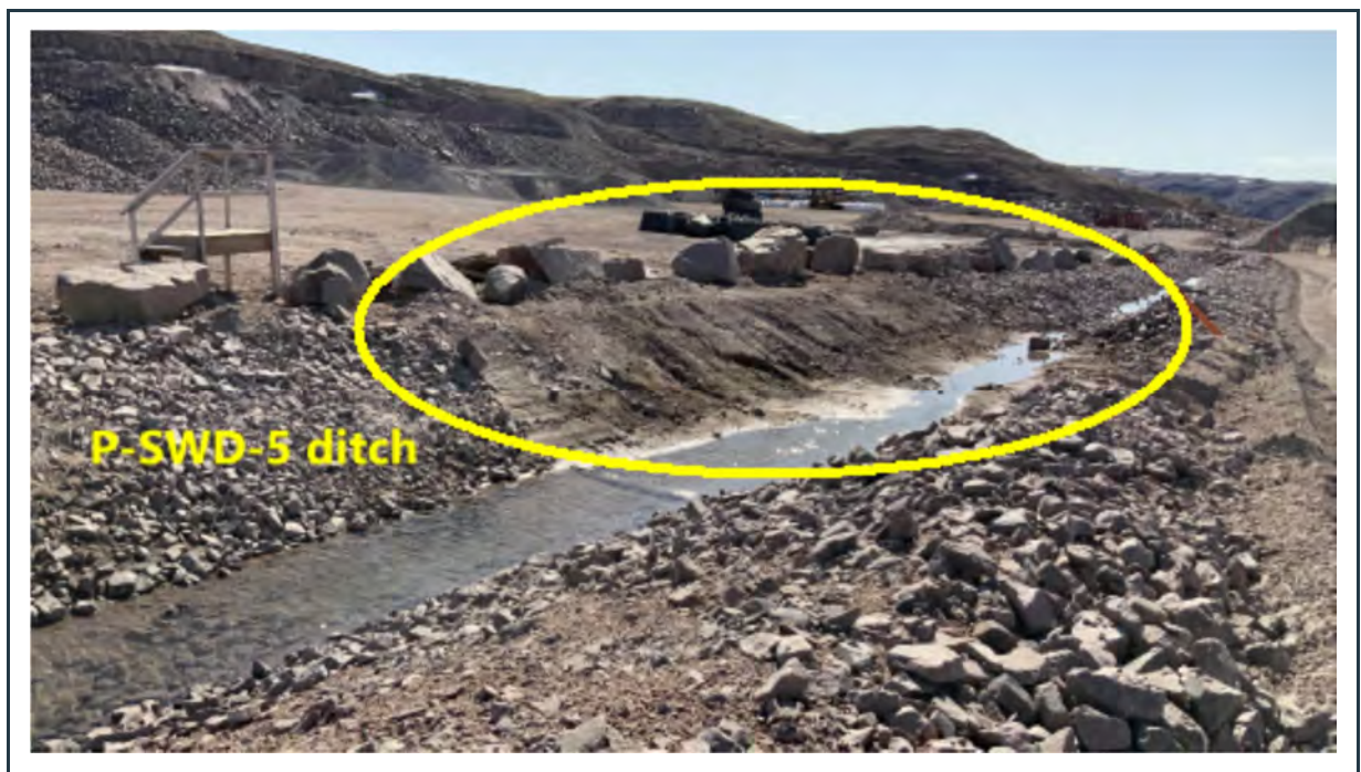
Figure 63: P-SWD-5 – “Q01-North” surface water collection ditch with missing riprap at one section of the ditch. Note the continuous seepage from the granular fill pad of the quarry’s lower (main) level.
