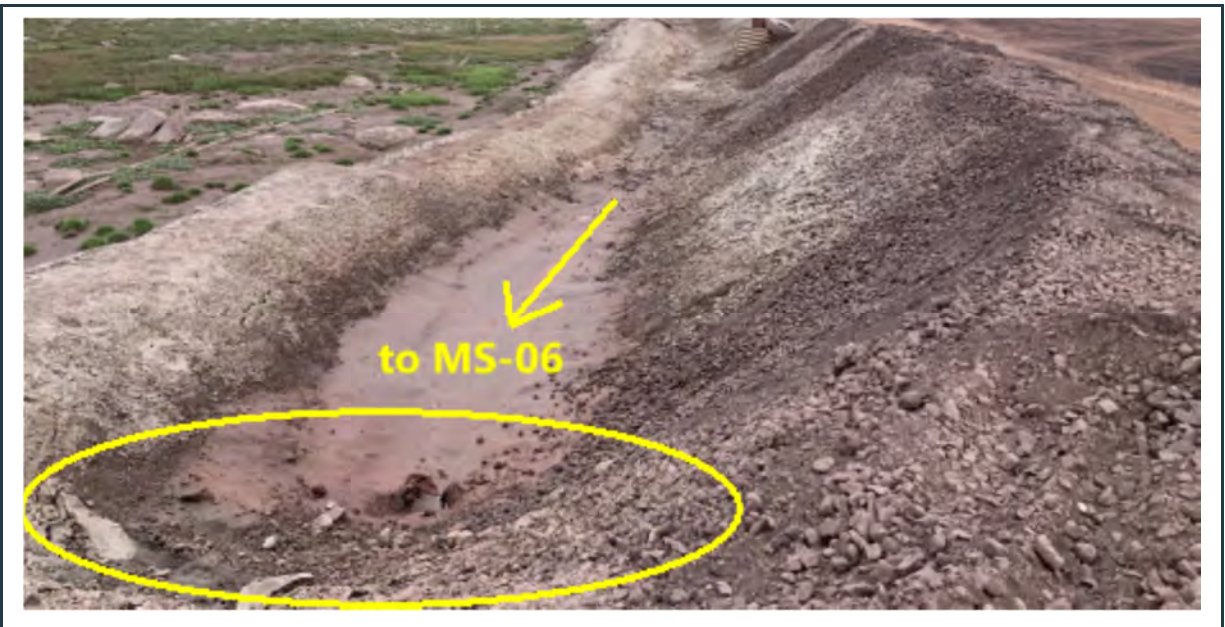
Figure 25: View of the partially clogged intake end of the culvert (yellow circle), shown in Figure 24. This end of the culvert should be cleaned as soon as practically possible.
