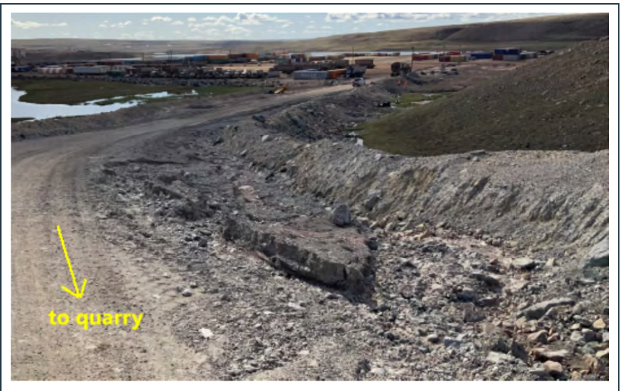
Figure 47: View of erosion related problems along the edge of the access road to the quarry.
