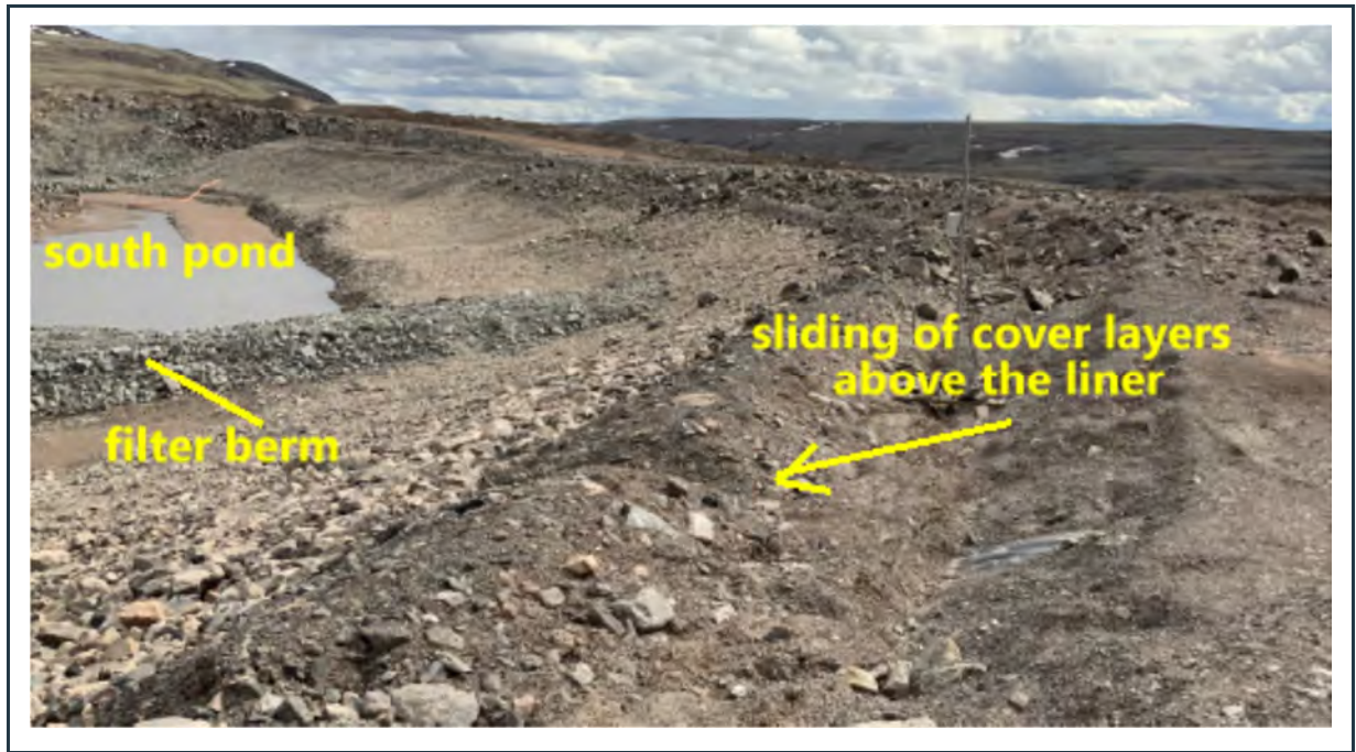
Figure 36: View of the new filter berm and sliding of the cover layers above the liner in the MS-11 south pond (image was taken in July 2025). See Figure 5 for the location of the new filter berm within the south pond.
