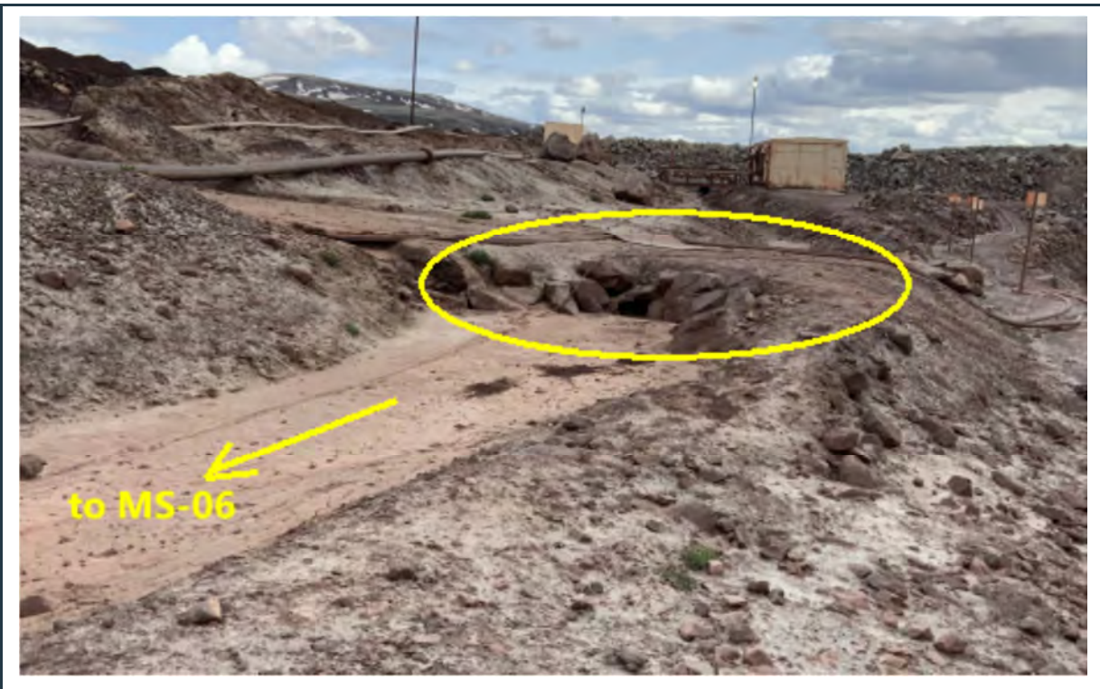
Figure 27: View of one of the side-ditches and a culvert leading to the MS-06 pond. As shown by the yellow circle, the culvert is damaged and clogged and should be replaced. Alternatively, the culvert could be removed permanently and the ditch opened for easy flow. See culvert B in Figure 2 for location.
