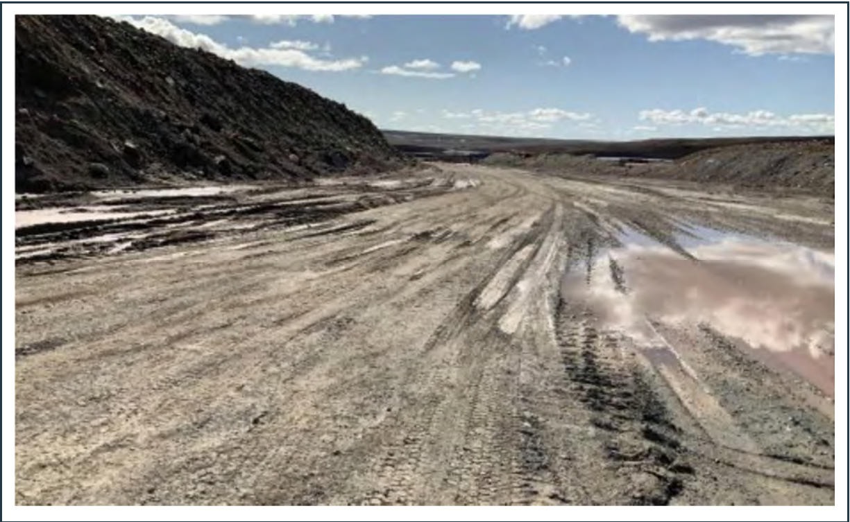
Figure 46: Drainage problems still exist at the first quarry level. Surface drainage shall be rectified.
