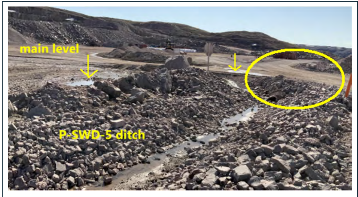
Figure 62: Poor surface water control in many areas of the lower (main) level of the Q01 rock quarry. The culvert at the entrance to the quarry (yellow circle) must be replaced.
