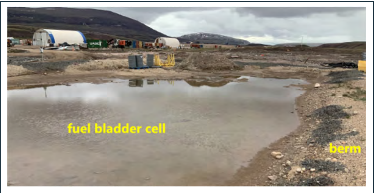
Figure 38: View of the stable perimeter berm around the practically empty “fuel bladder” cell. Note only three grey fuel barrels at the corner of the cell. The ponding water in the cell indicates good liner performance.
