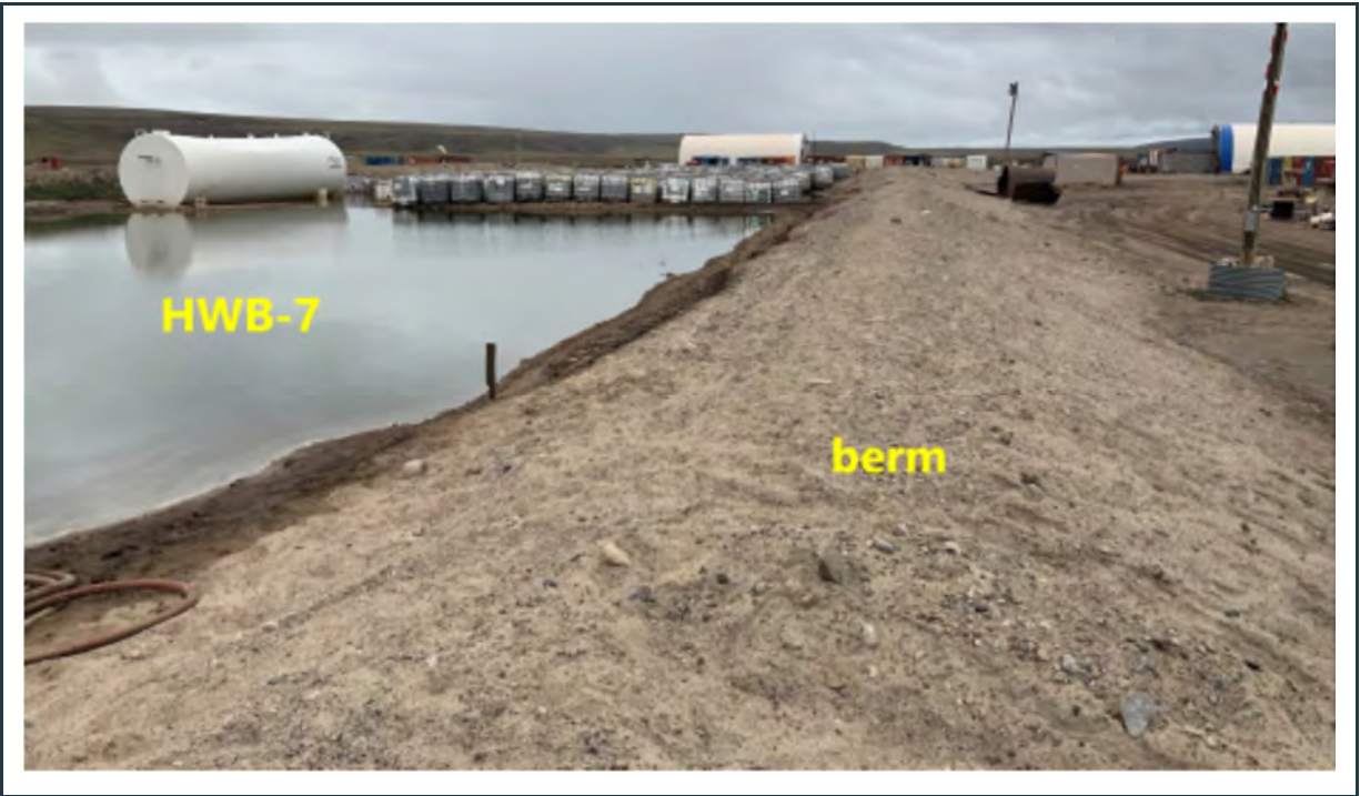
Figure 22: View of the stable berm around the HWB-7 cell, with an old fuel tank and oil filled plastic containers stored in the cell. The ponding water indicates good liner performance.
