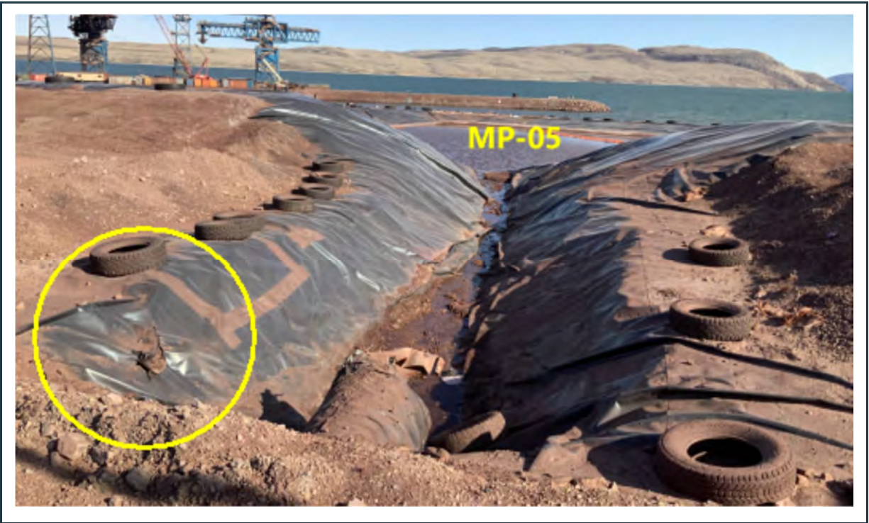
Figure 58: View of the slightly damaged liner (yellow circle) at the intake channel to the MP-05 pond.
