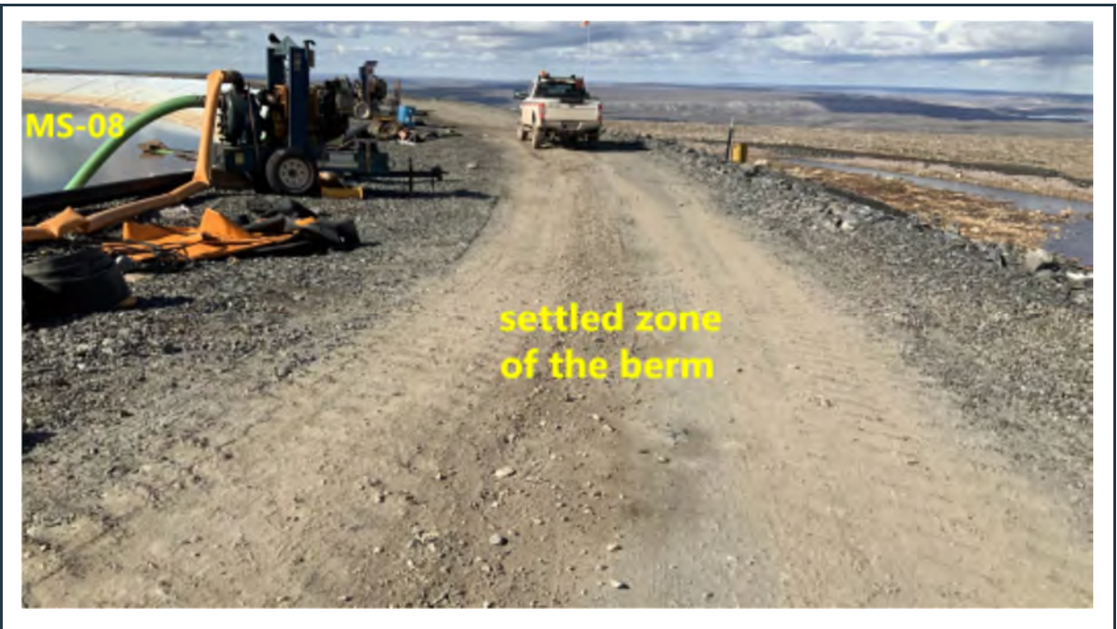
Figure 30: View of a settled zone of the berm, where two pumps are located. The anchor trench of the liner is still in its original position. The crest of the berm along this zone should be raised to its original crest elevation by crushed aggregate.
