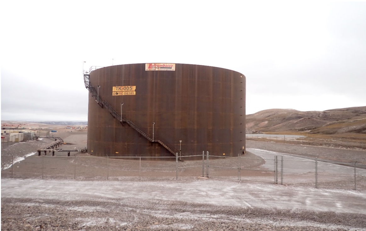
Photo 48. Mine Site Bulk Fuel Storage Facility (MS-03B) - August
