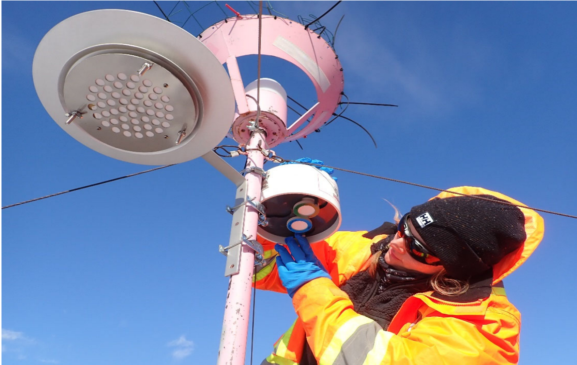
Photo 87. Passive NOx and SOx Monitoring Filter Installation at Remote Site – September
