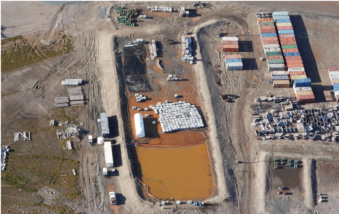
Photo 71. Oily Waste Water Treatment at Hazardous Waste Berm 7 – August
