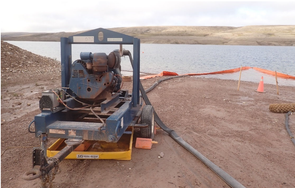
Photo 10. KM 32 Water Withdrawal Pump at Katiktok Lake - August
