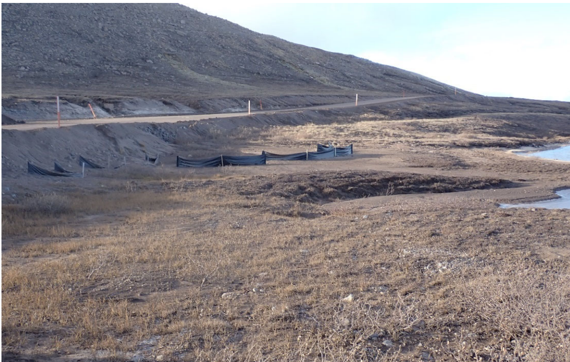
Photo 46. Erosion and Sediment Control Silt Fence at KM 87.5 Water Crossing (BG-24) – September
