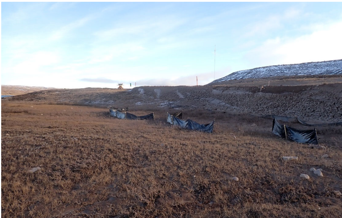
Photo 47. Erosion and Sediment Control Silt Fence at KM 87.5 Water Crossing (BG-24) – September
