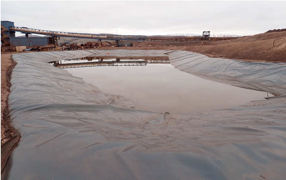
Photo 5. Surface Water Management Pond (MP-06A), Southwest Cell of Ore Stockpile Pad– September
