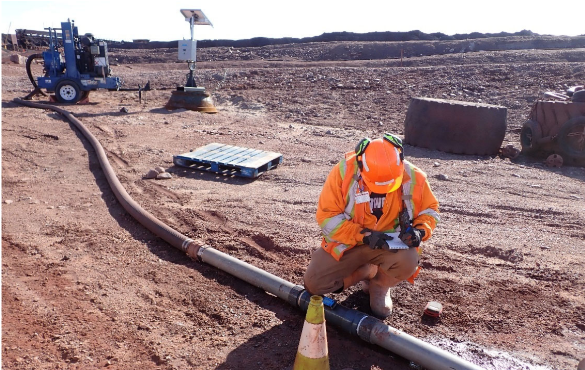
Photo 13. Discharge Monitoring at Surface Water Management Pond (MP-06A) – August
