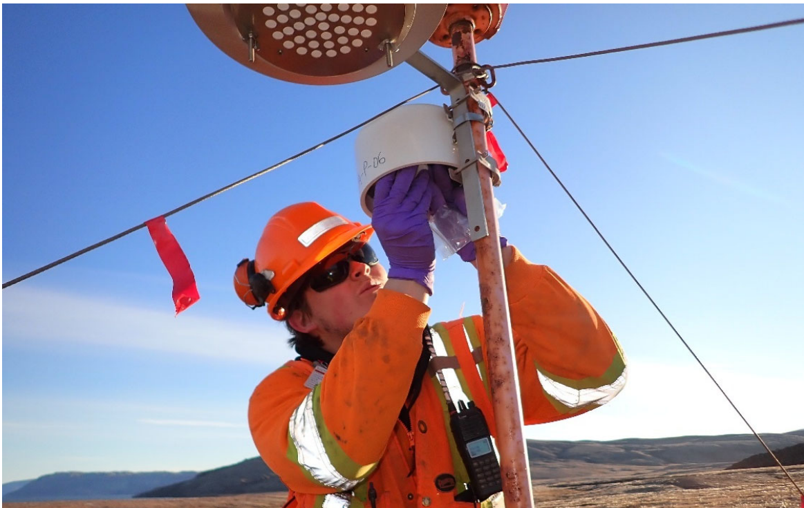
Photo 32. Passive NO x and SO x Monitoring Filter Installation (PA-P-06) – September
