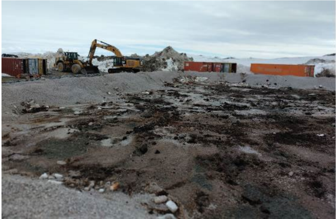
Photo 3. Geotube® removed and liner damaged – June 21
