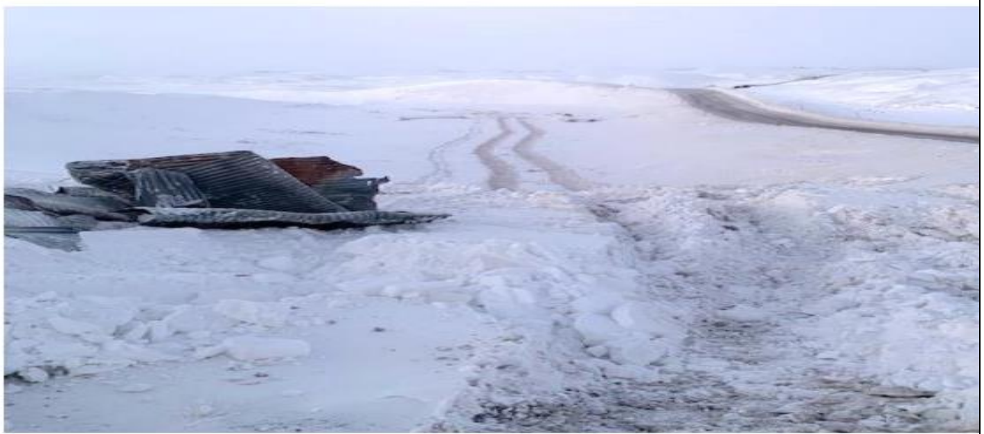
Photo 4. KM 63.5, Culverts retrieved from watercourse, staged next to Tote Road for pick final disposal, 2024-11-28
