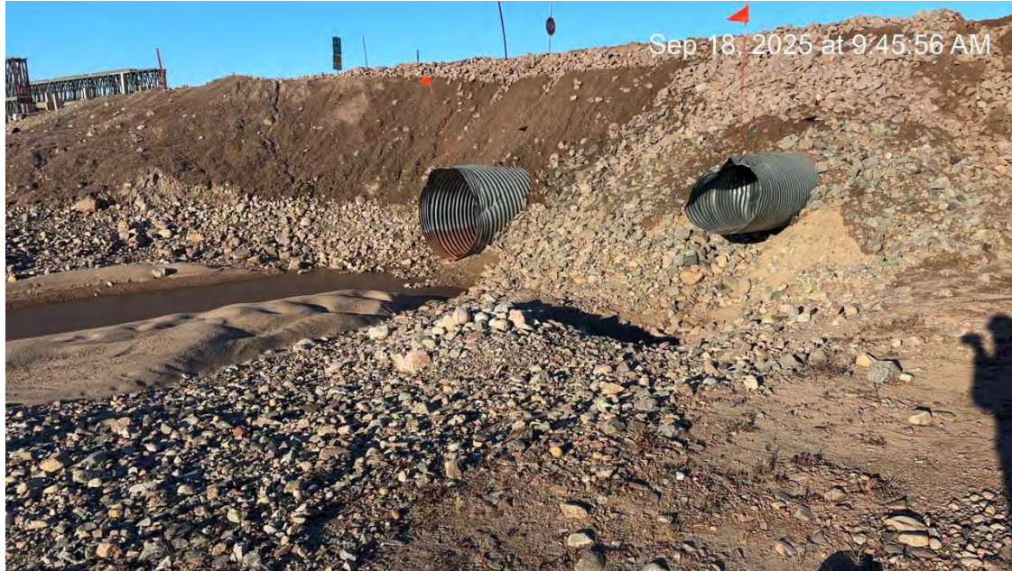
Photo 27 – Perched culverts at KM97 (September 18, 2025).
