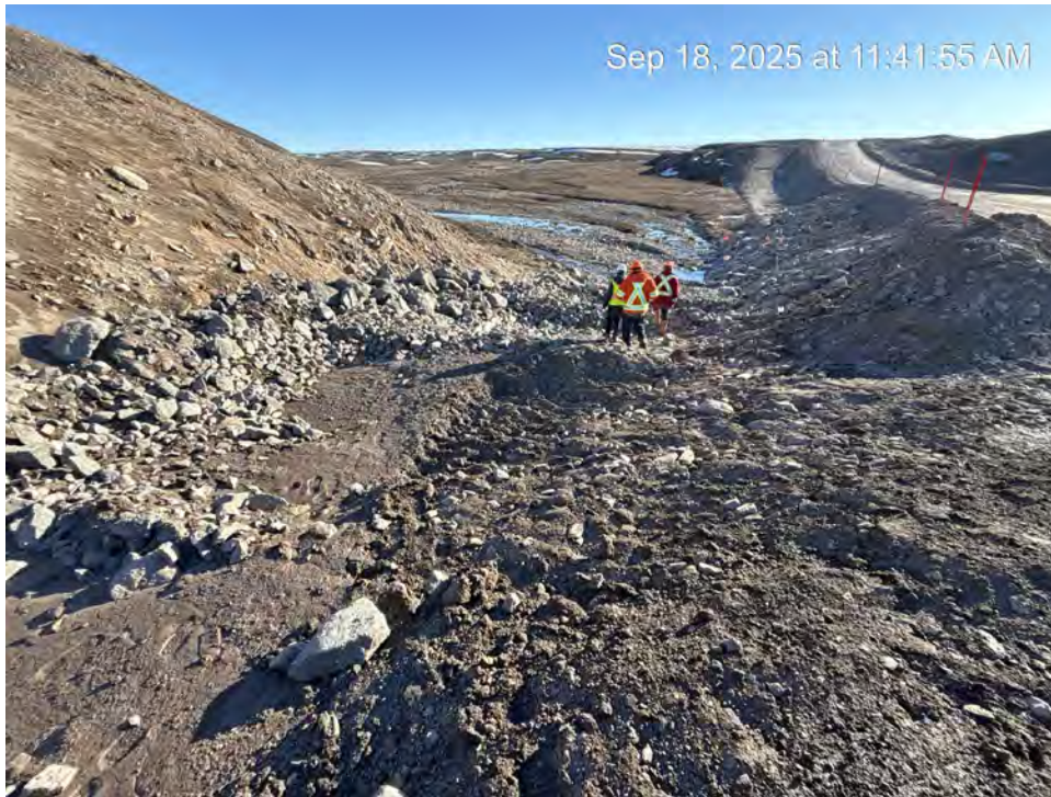
Photo 41 –Accumulation of sediment in check dams at KM64 (September 18, 2025).
