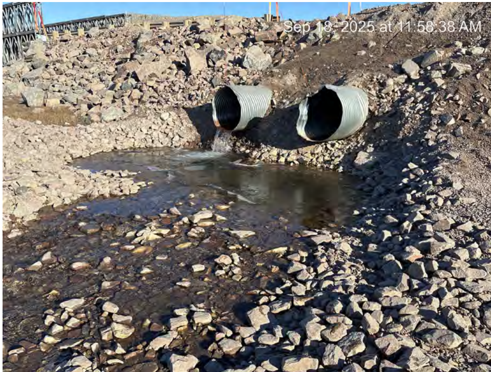
Photo 45 – Perched culverts at KM63 bridge (September 18, 2025).
