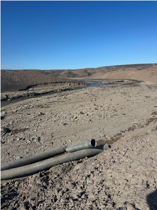
Photo 24 – Culverts still scattered at KM63.5 (June 19 th , 2025).
