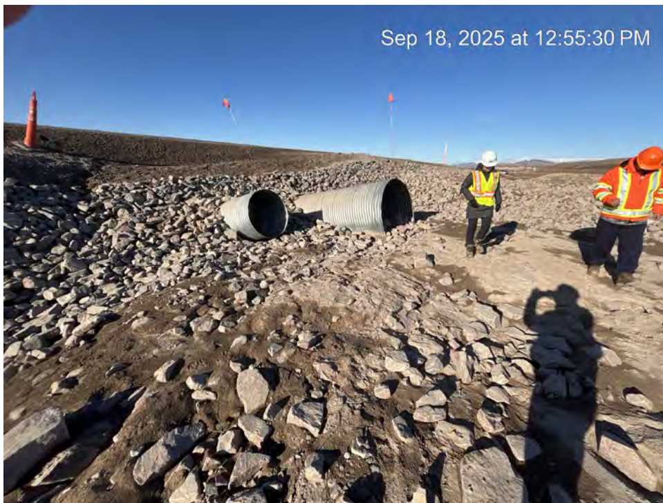
Photo 48 – Blocked culverts at KM33 (September 18, 2025).
