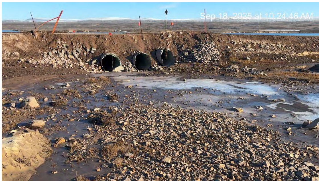
Photo 34 – Culverts to be replaced at KM87.5 (September 18, 2025).
