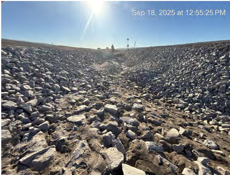
Photo 47 – Sediment accumulation but no flow in ditch upstream of culverts at KM33 (September 18, 2025).
