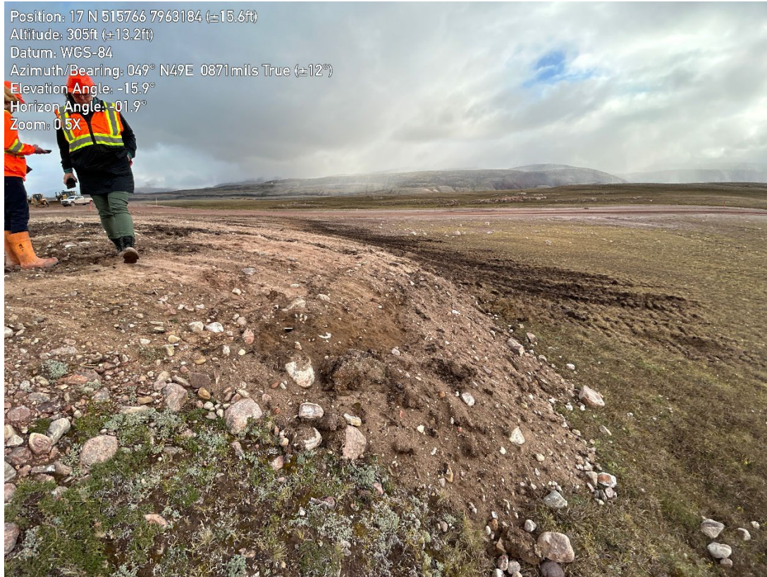
Figure 3.14: Edge of reclaimed borrow area at KM 37, placed at relatively steep slope.
