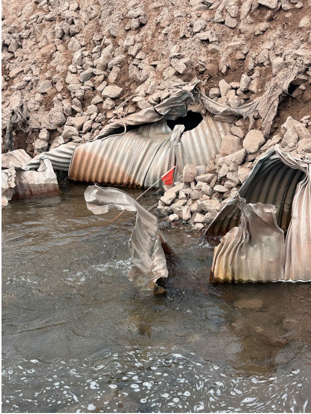
Photo 15 – Damaged culverts behind Sailiivik Camp (June 18 th , 2025).
