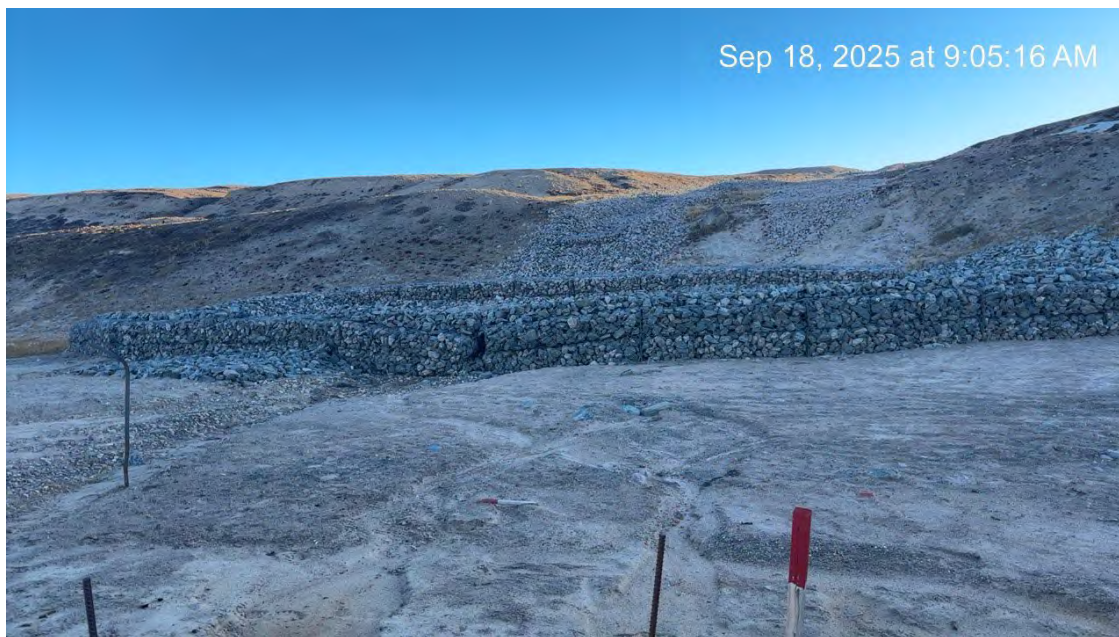
Photo 22 – Gabion wall at Camp Lake (September 18, 2025).
