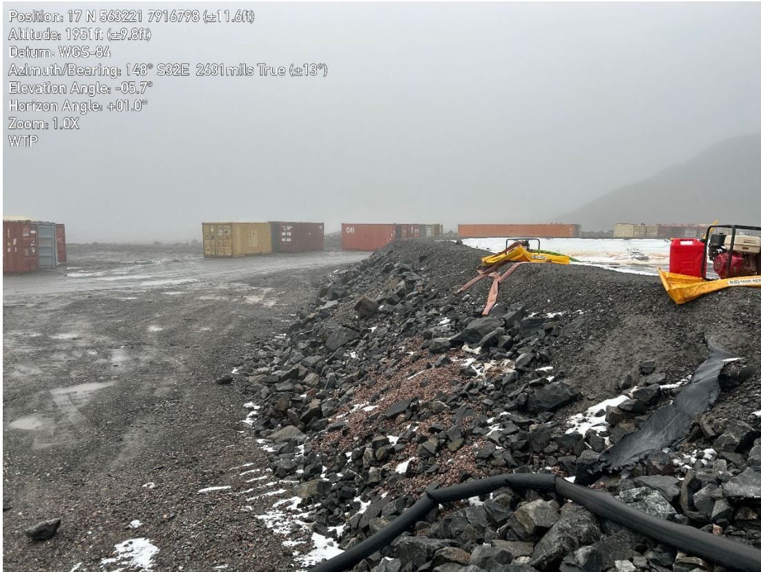
Figure 3.4: Water treatment plant containment berms
