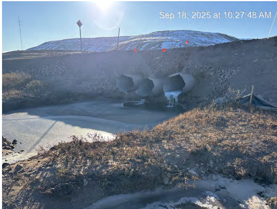
Photo 35 – Perched culverts and erosion on embankment at KM87.5 (September 18, 2025).
