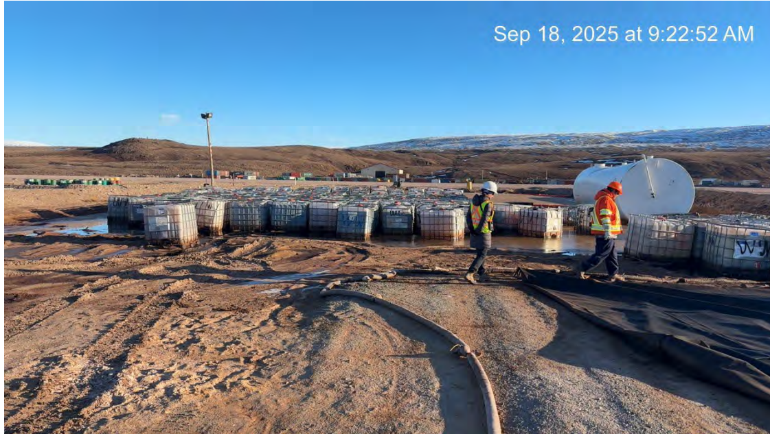
Photo 25 – Labelled totes at Oil Water Separator (September 18, 2025).
