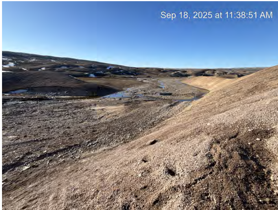
Photo 43 – Location of washed-out culverts at KM64 that need to be removed (September 18, 2025).
