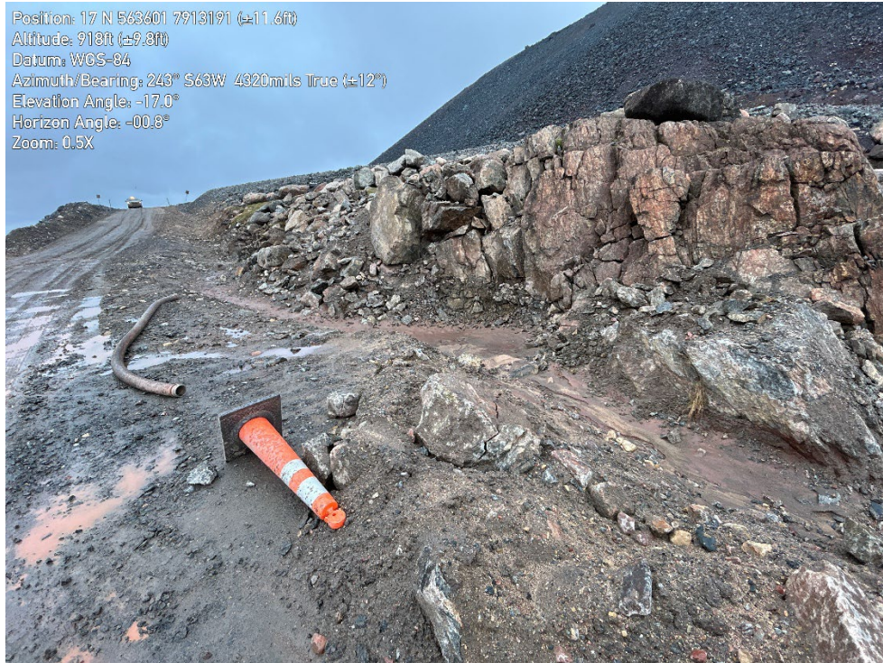
Figure 3.7: Uncontrolled seepage from KM 106 pumped to MS-07 sediment pond.
