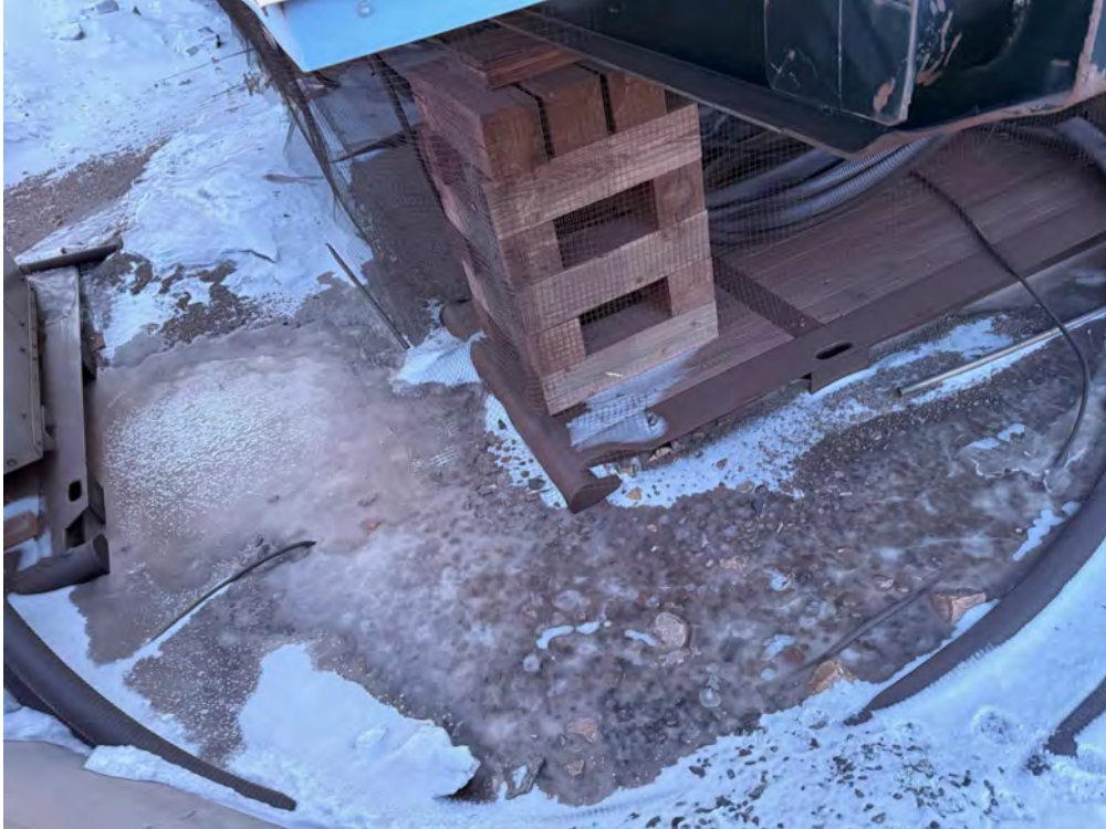
Photo 3: Mine Site Complex Laundry Lift Station Spill Location – Spilled Sewage Frozen on Ground Near Transformer - March 29, 2025
