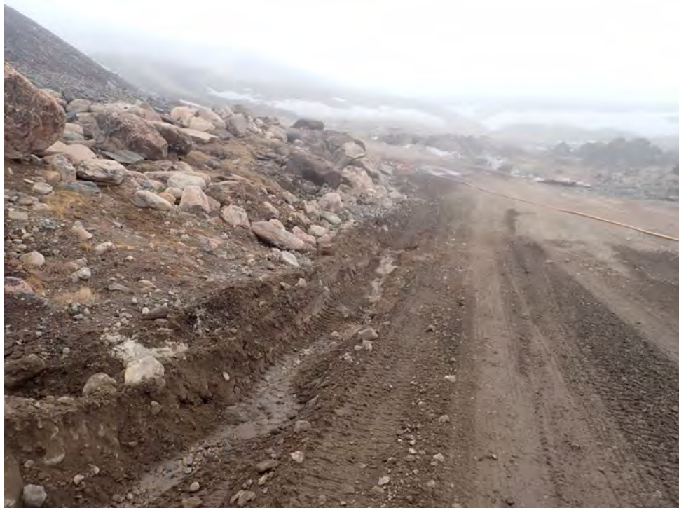
Photo 4: Ditch Maintained to Intercept/Redirect Seepage to Existing Containment Sump – June 7, 2025
