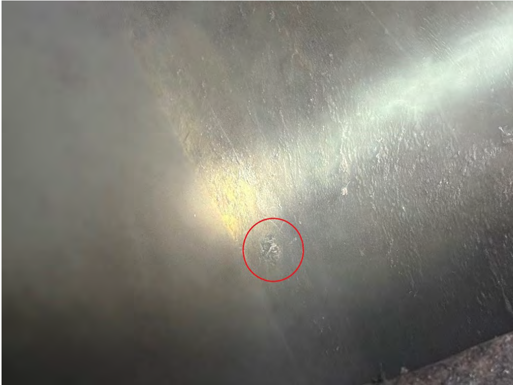
Photo 5: Mine Site Complex Laundry Lift Station – Crack in the tank - March 29, 2025
