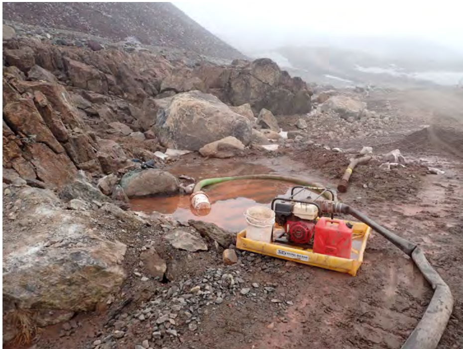
Photo 5: Existing Containment Sump, with Pump Infrastructure in Place to Transfer Water to the MS-07 Containment Pond – June 7, 2025
