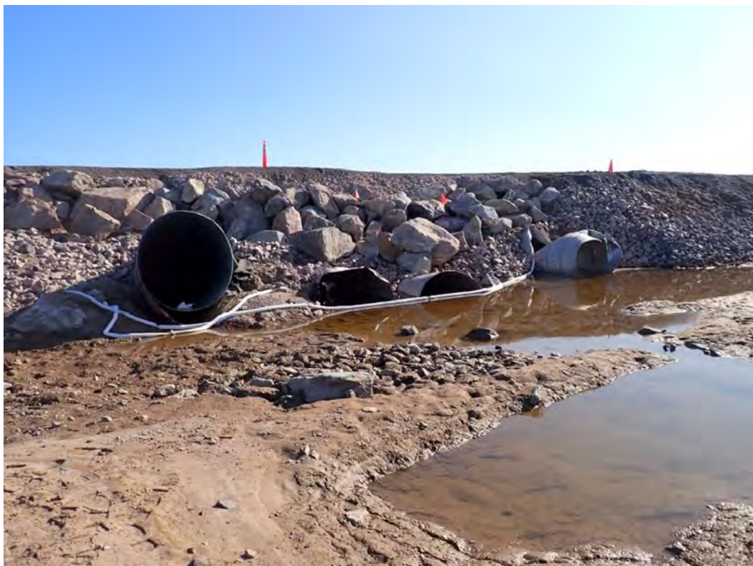
Photo 6: Upstream Conditions Prior to Removal of Spill Response Equipment – July 20, 2025
