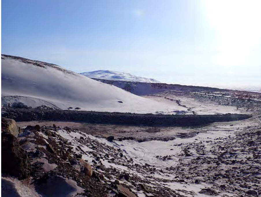
Photo 1. Filter Berm within KM 105 Valley Water Management Infrastructure – March 31, 2025
