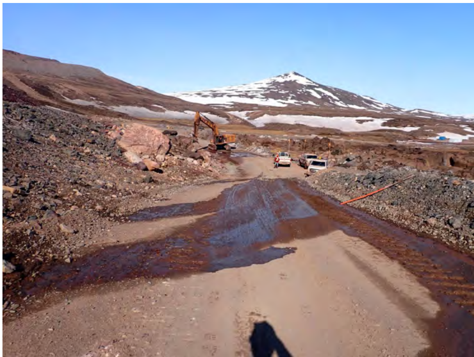
Photo 2: Seepage Location, Adjacent to the MS-07 Containment Pond – June 6, 2025
