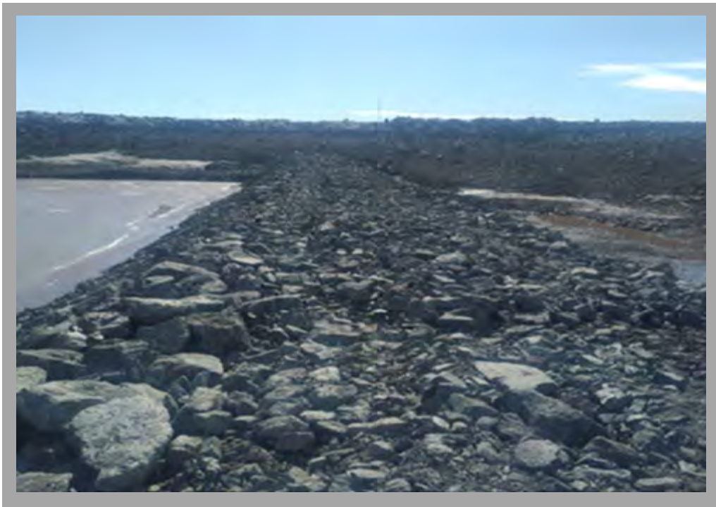
Photo 8: Filter Berm operating within Km 105 valley infrastructure above SDLT- May 23 rd 2025
