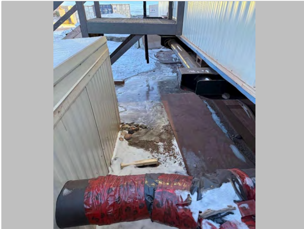
Photo 2: Mine Site Complex Laundry Lift Station Spill Location – Spilled Sewage Frozen on Ground - March 29, 2025
