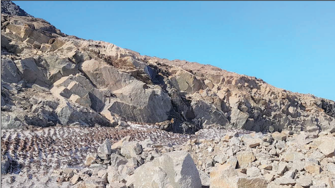
PHOTO 4 – Upper Quarry Area - Seep at eastern end of wall
