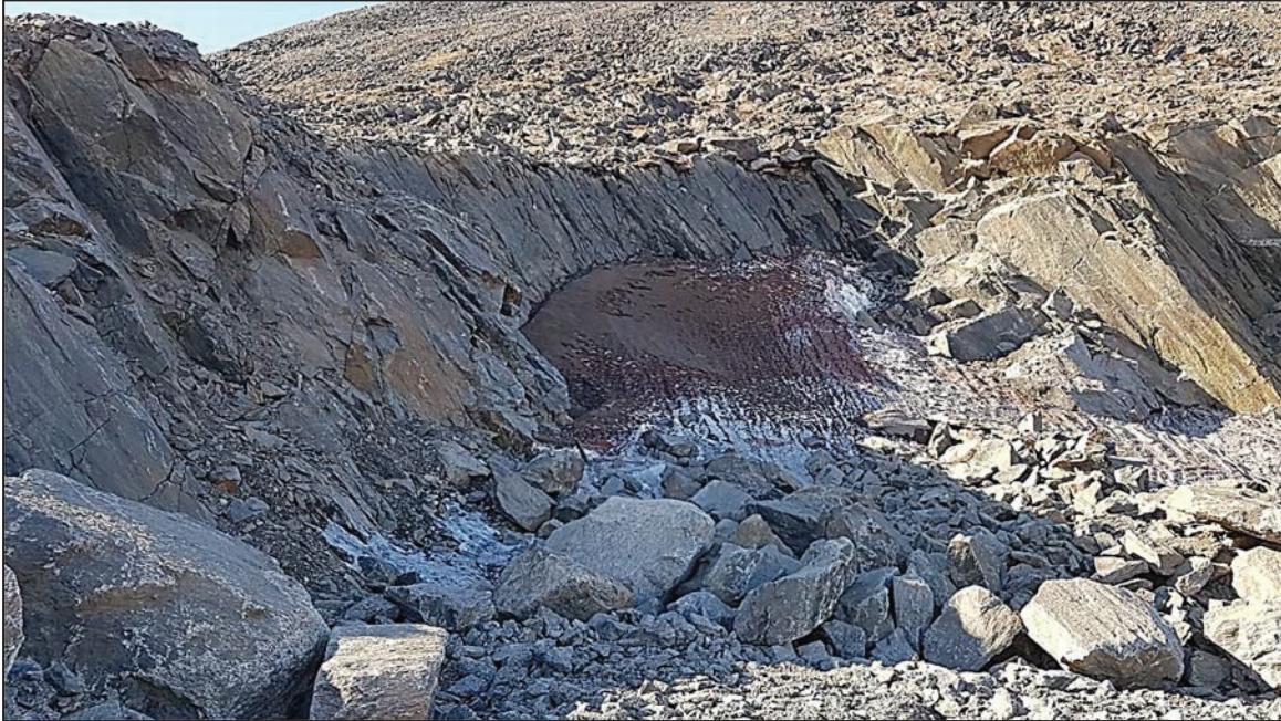
PHOTO 3 – Upper Quarry Area - Loose blocks at crest and accumulated at toe
