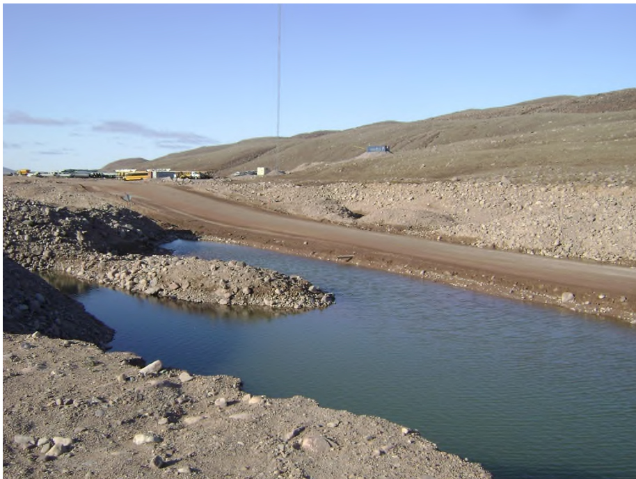
Photo 7 (2531): Pit at KM 7.2 with water on both sides of the new road alignment and extensive thaw of massive and wedge ice.
