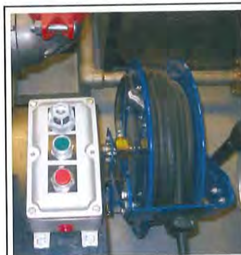
Lube oil control
