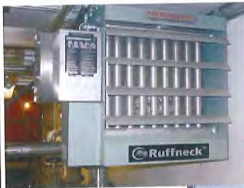
Fueling area heater
