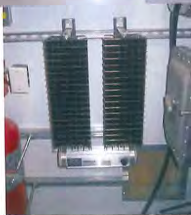
Electrical room heaters
