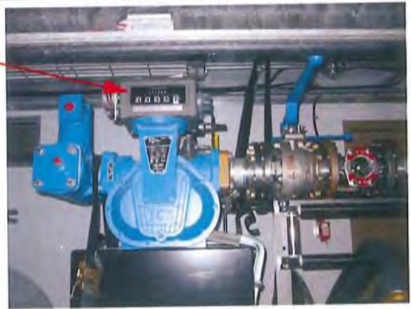
Tanker truck fuel meter
