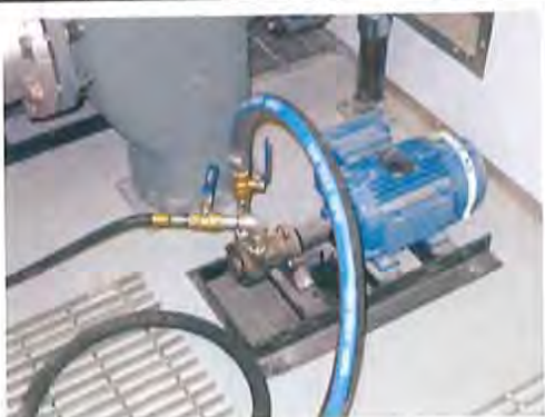
The lube oil pump is installed near the tote tank.
