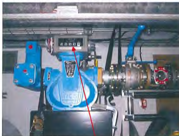
Tanker truck fuel meter
