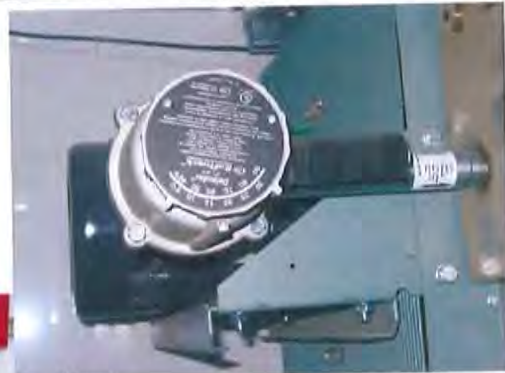
Fueling area thermostat
