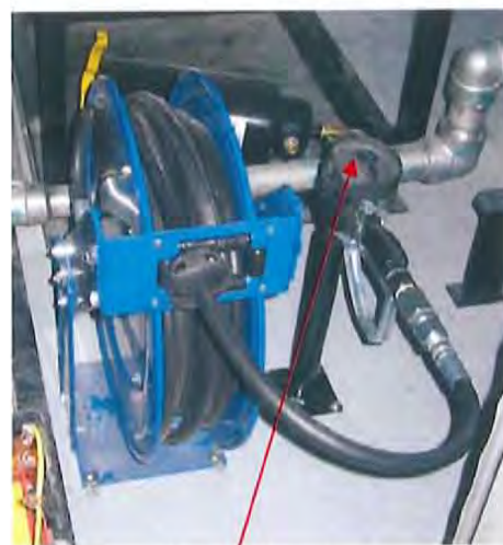
Lube oil meter
