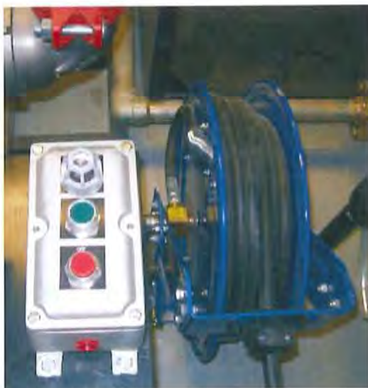
Lube oil control
