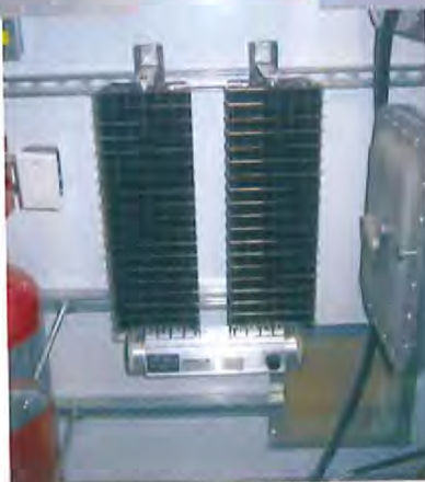
Electrical room heaters
