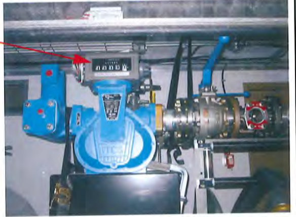
Tanker truck fuel meter
