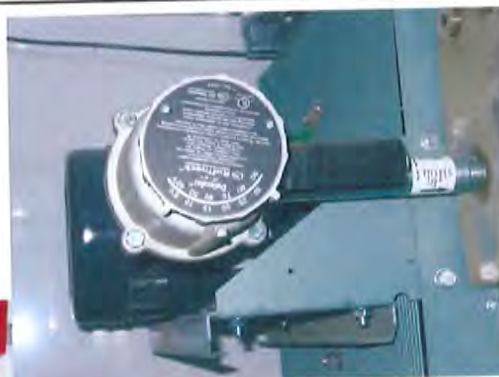
Fueling area thermostat
