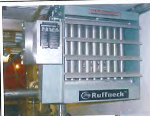
Fueling area heater
